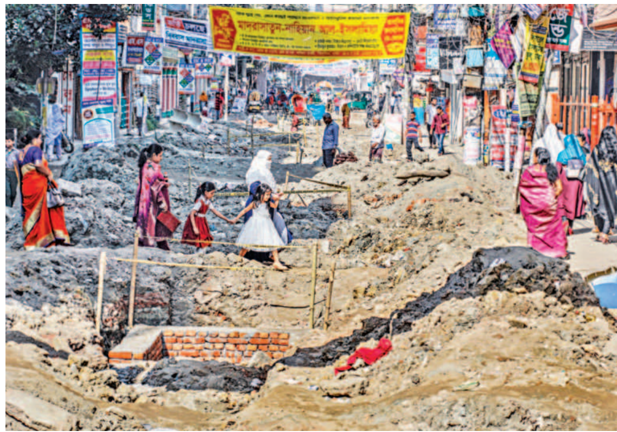
The city corporations are installing sewage lines in South Banasree road at a snail's pace. Locals have been putting up with the dug-up road for almost a year now. The photo was taken yesterday. PHOTO: RASHED SHUMON
