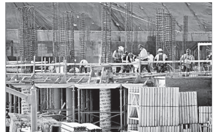
Work crews construct a new hotel complex on oceanfront property in Encinitas, California on November 27.
