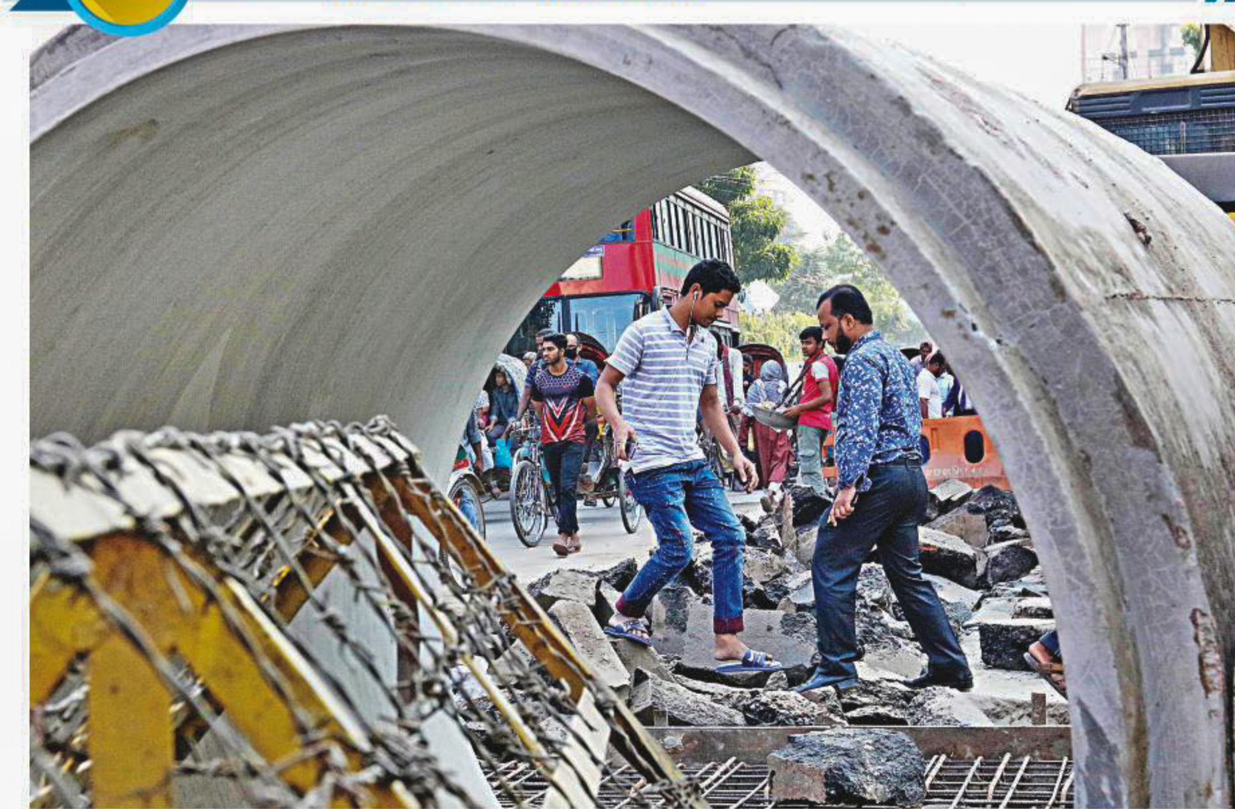
Pedestrians have to calculate risks, then perform some careful acrobatics to walk on the Dainik Bangla intersection, which was dug up three months ago to install sewage lines. Traffic police stationed at the area also complained that controlling vehicle movement has become a difficult task.
