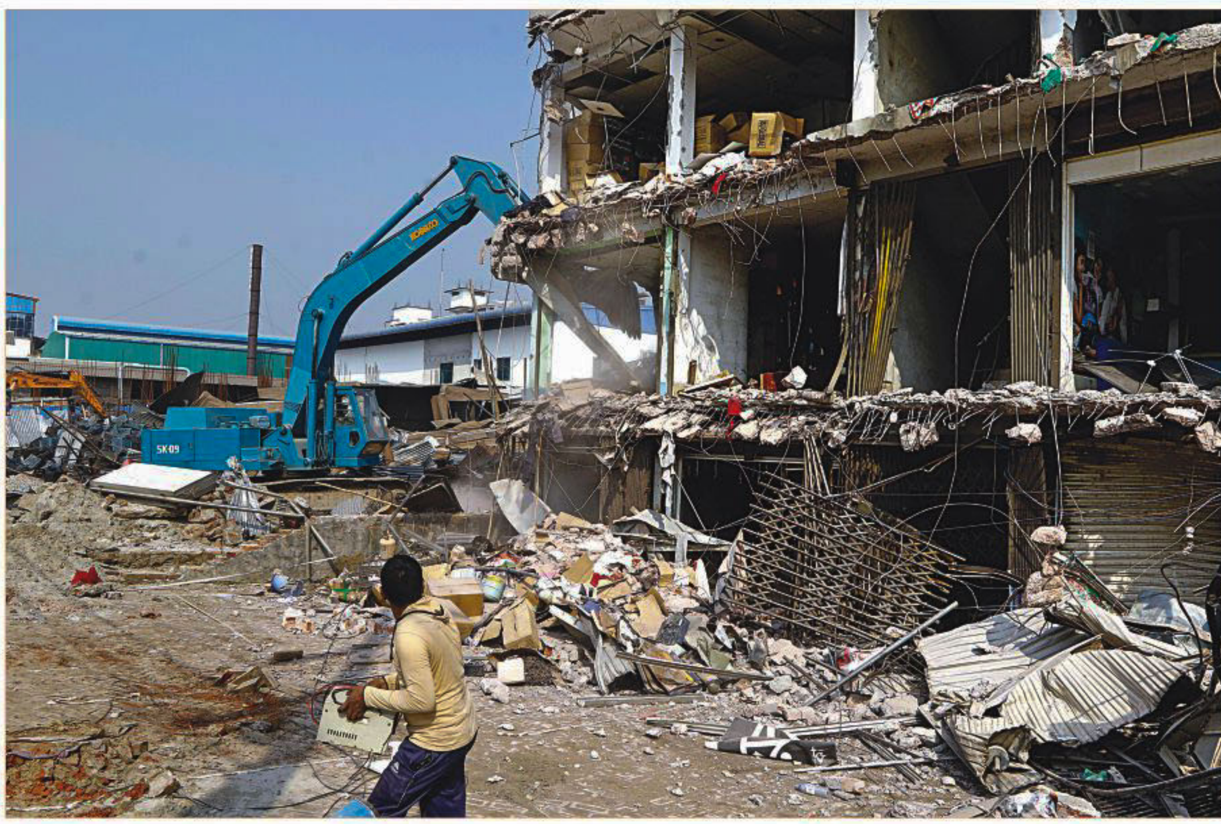
A bulldozer knocks down a part of a market building on the Dhaka-Aricha highway in Savar Thana Stand area yesterday during a drive by Roads and Highways Department against illegal structures.
