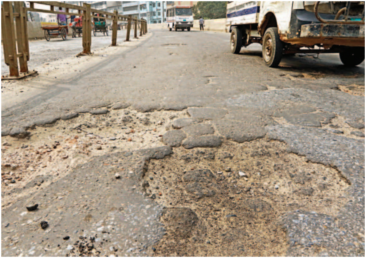
With worn-out surface and potholes at numerous spots, commuters are always in for a bumpy ride on Babubazar bridge in Old Dhaka. The photo was taken recently.
