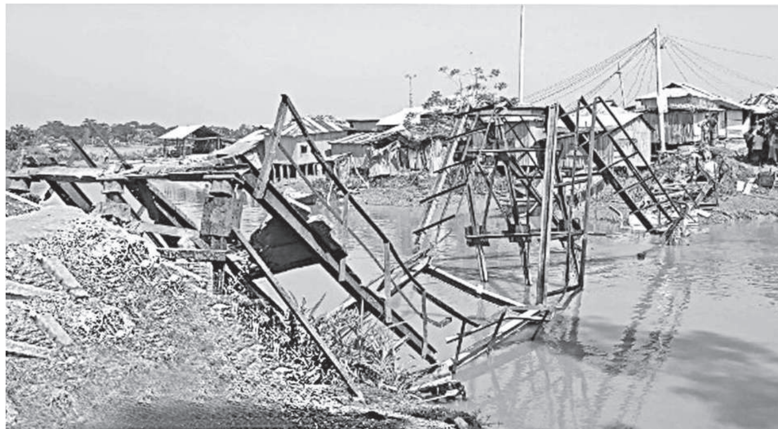
The iron bridge on a canal has been lying collapsed for a week, causing immense sufferings to people of six villages in Patuakhali's Kalapara upazila.
