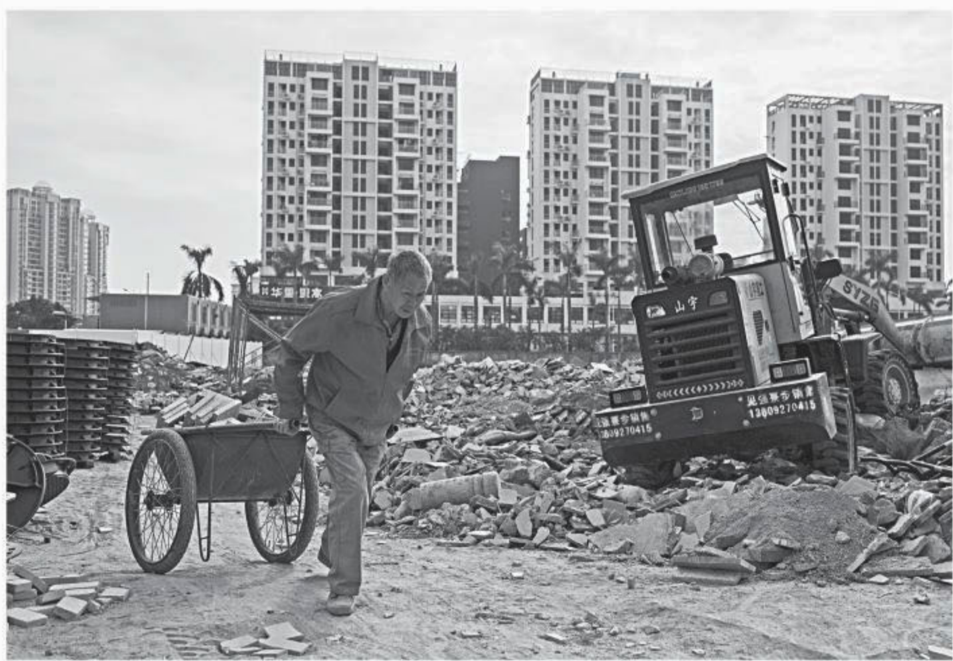
A worker pulls a cart at a construction site in the Shekou area of Shenzhen, China.
