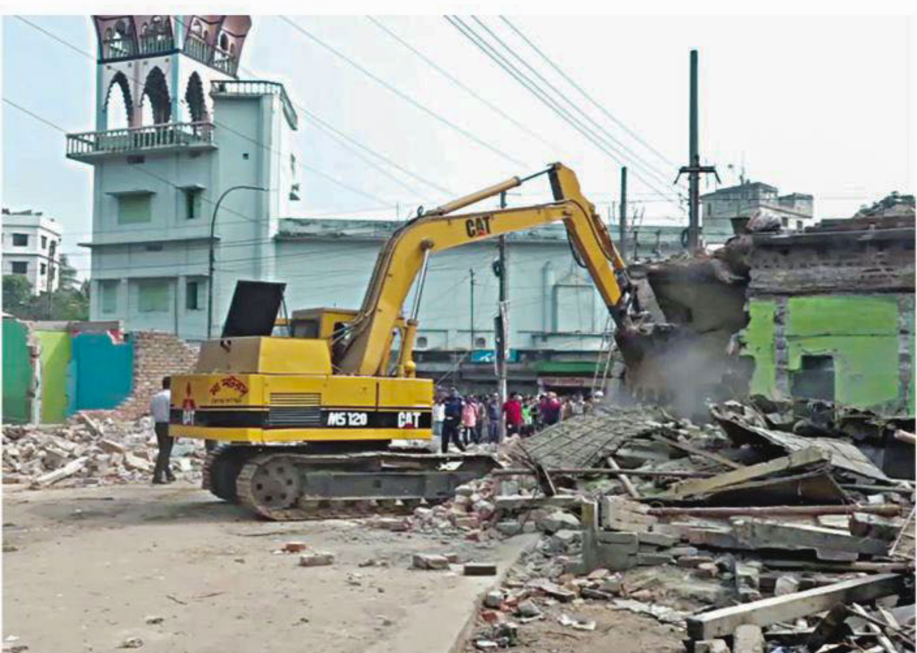
Illegal structures on the premises of Mymensingh railway station being torn down during a drive by railway authorities. The photo was taken on Tuesday.
