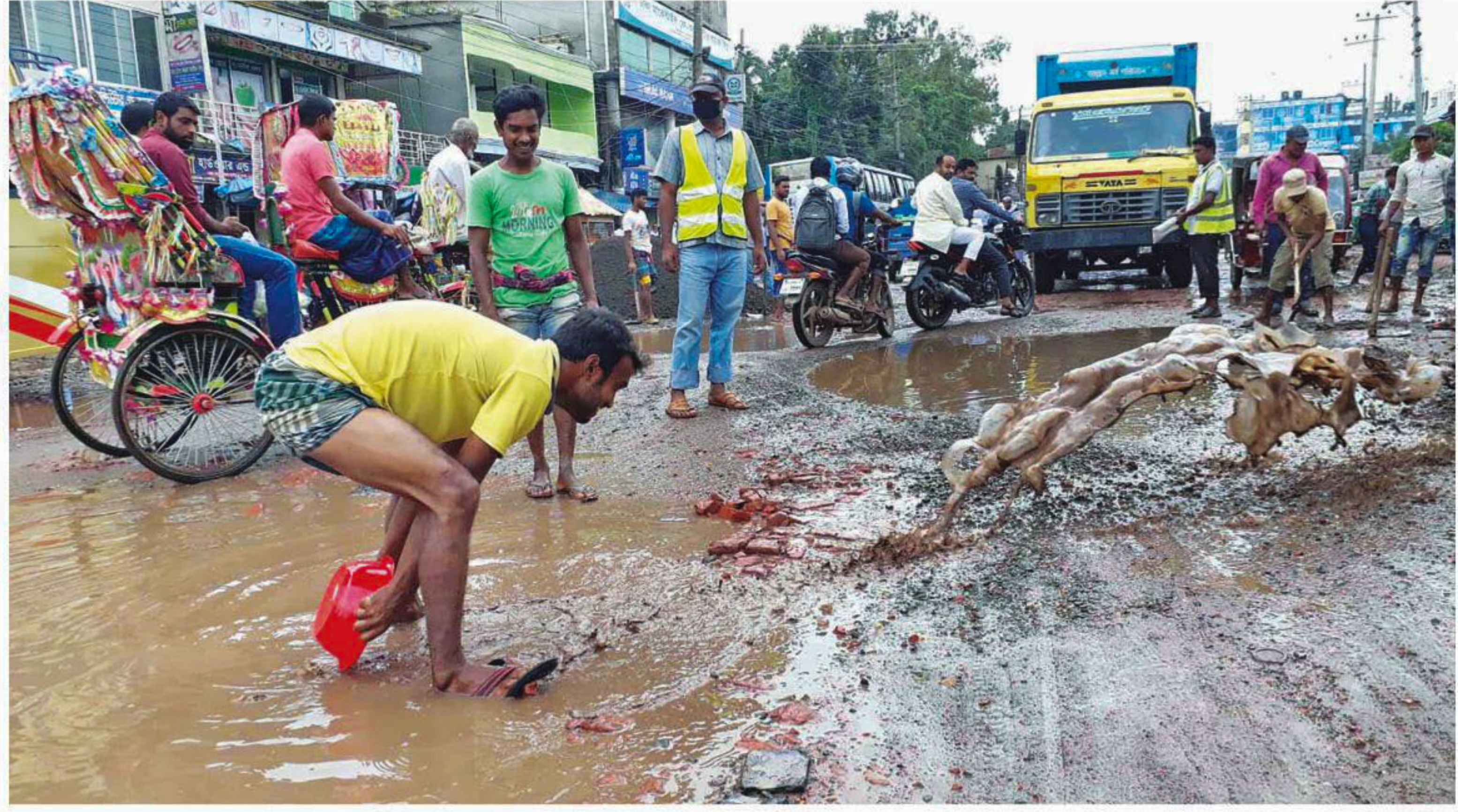
Without any proper equipment provided for the task, a worker uses a household bowl to scoop out water from a large pothole near Ghatail bus stand on the Elenga-Jamalpur highway, being converted into four lanes. People are being subjected to health hazards as well as rampant accidents on the highway as the contractors are not following standard safety practices. The photo was taken recently.
