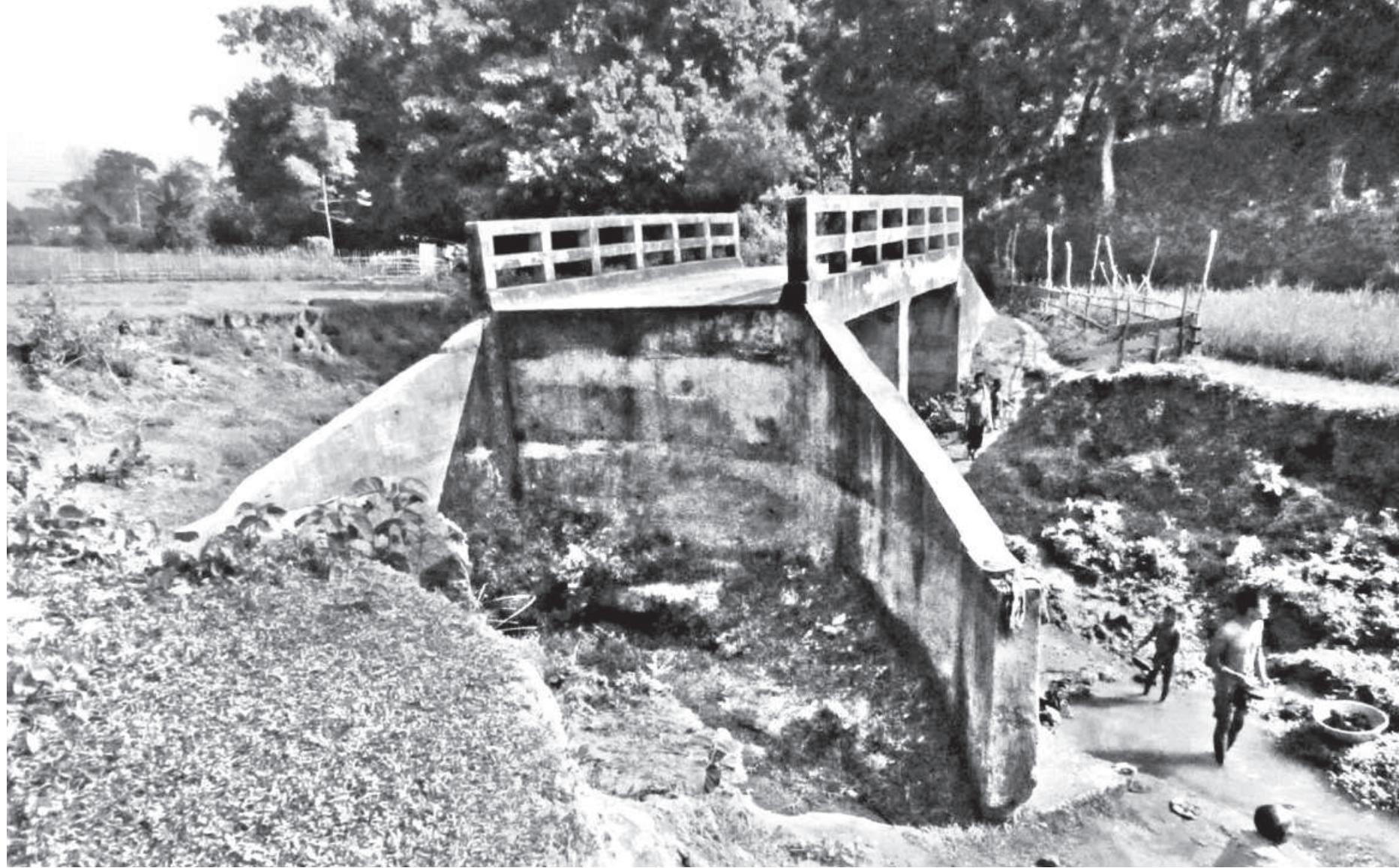
This culvert at West Golabari under Golabari union in Khagrachhari Sadar upazila fails to facilitate vehicular movement as the earthen road on either side have not been made usable for vehicles.
