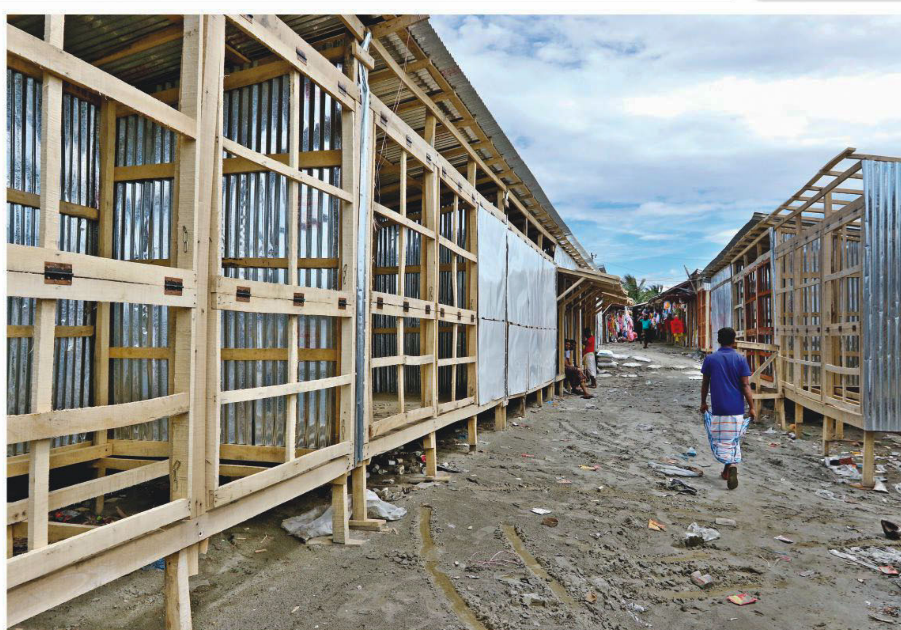
Rows of shops are being constructed illegally ahead of the tourist season on Kuakata beach in Patuakhali. The view on the wide-open beach gets ruined by these shops. Moreover, these shops are a major source of litter that diminish the joy of going to the beach. The photo was taken last week.
