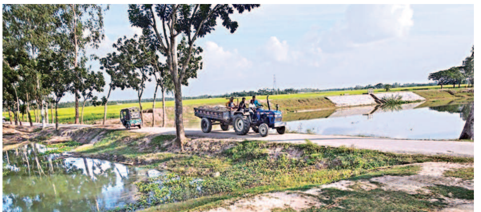
This road obstructs flow in Bogra major branch canal under Teesta Irrigation Project at Belaichondi village in Parbatipur upazila, thanks to the negligence of the authorities concerned.
