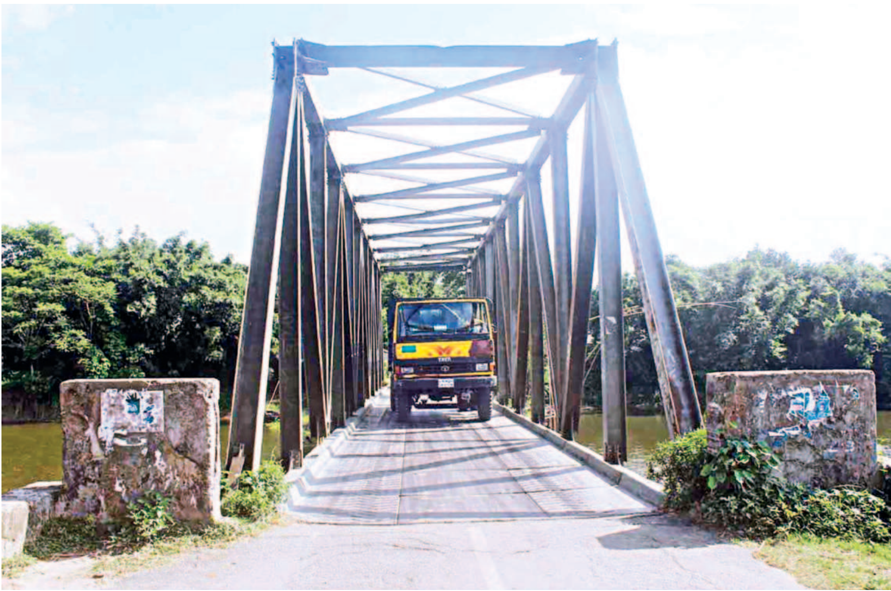
A ramshackle Bailey bridge on Tangail-Aricha road at Tirsra in Nagarpur upazila of Tangail.
