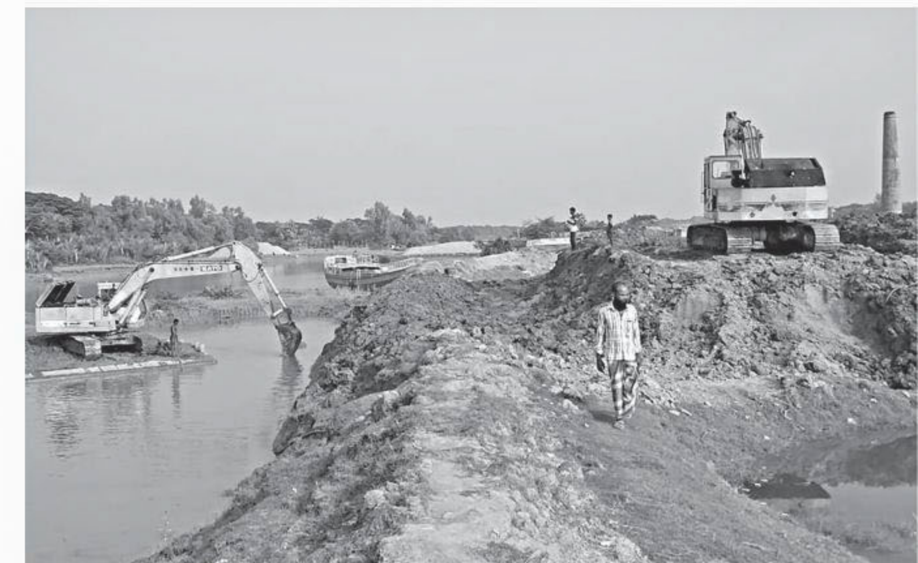
Local ruling party men cut earth illegally from the Shibbaria river with excavators in Patuakhali's Kalapara upazila. The photo was taken on Saturday.
