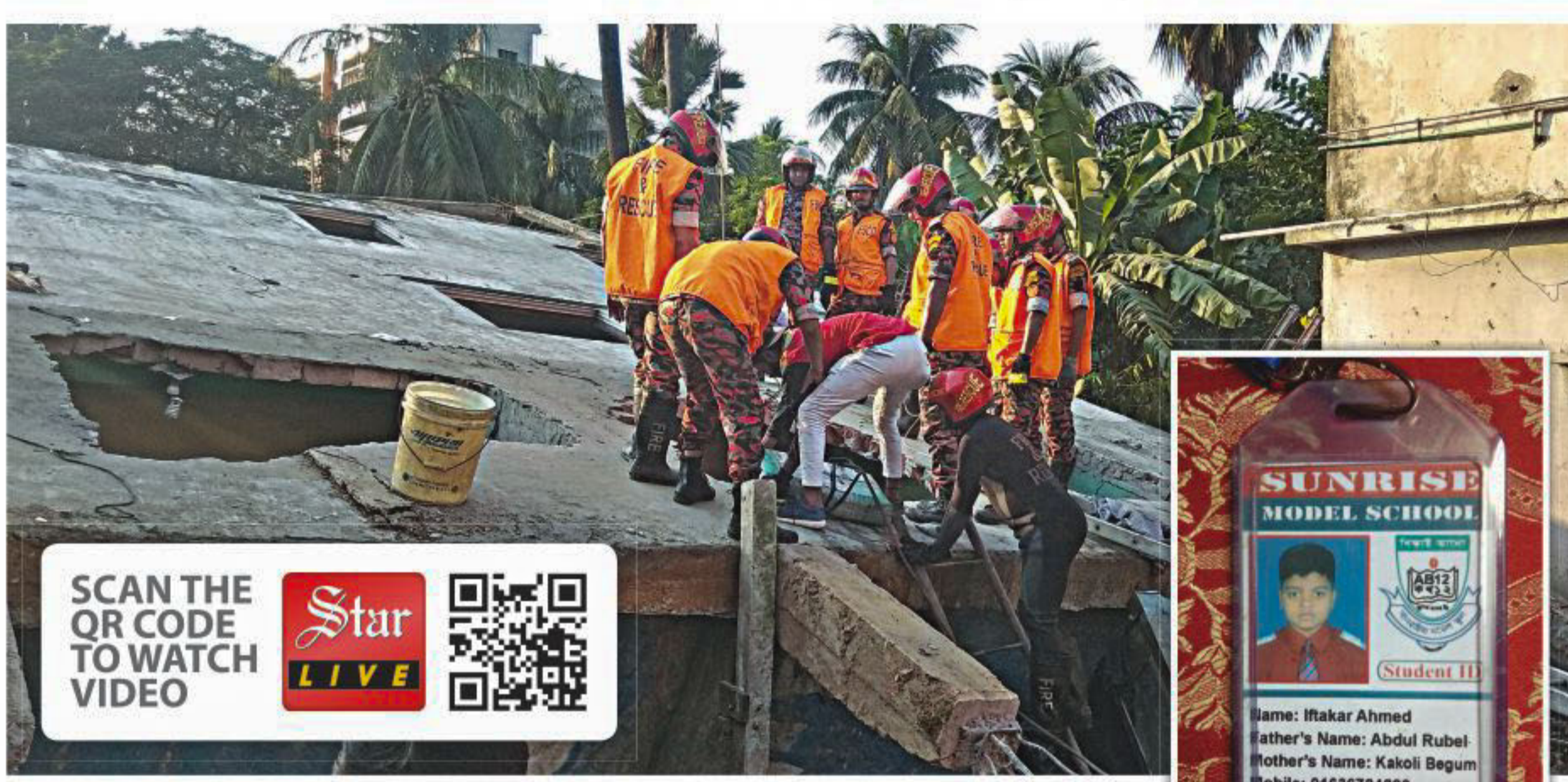
Fire service rescuers think Iftakar Ahmed Wazid, inset, might be trapped in the building corridor that has gone under water and mud.
