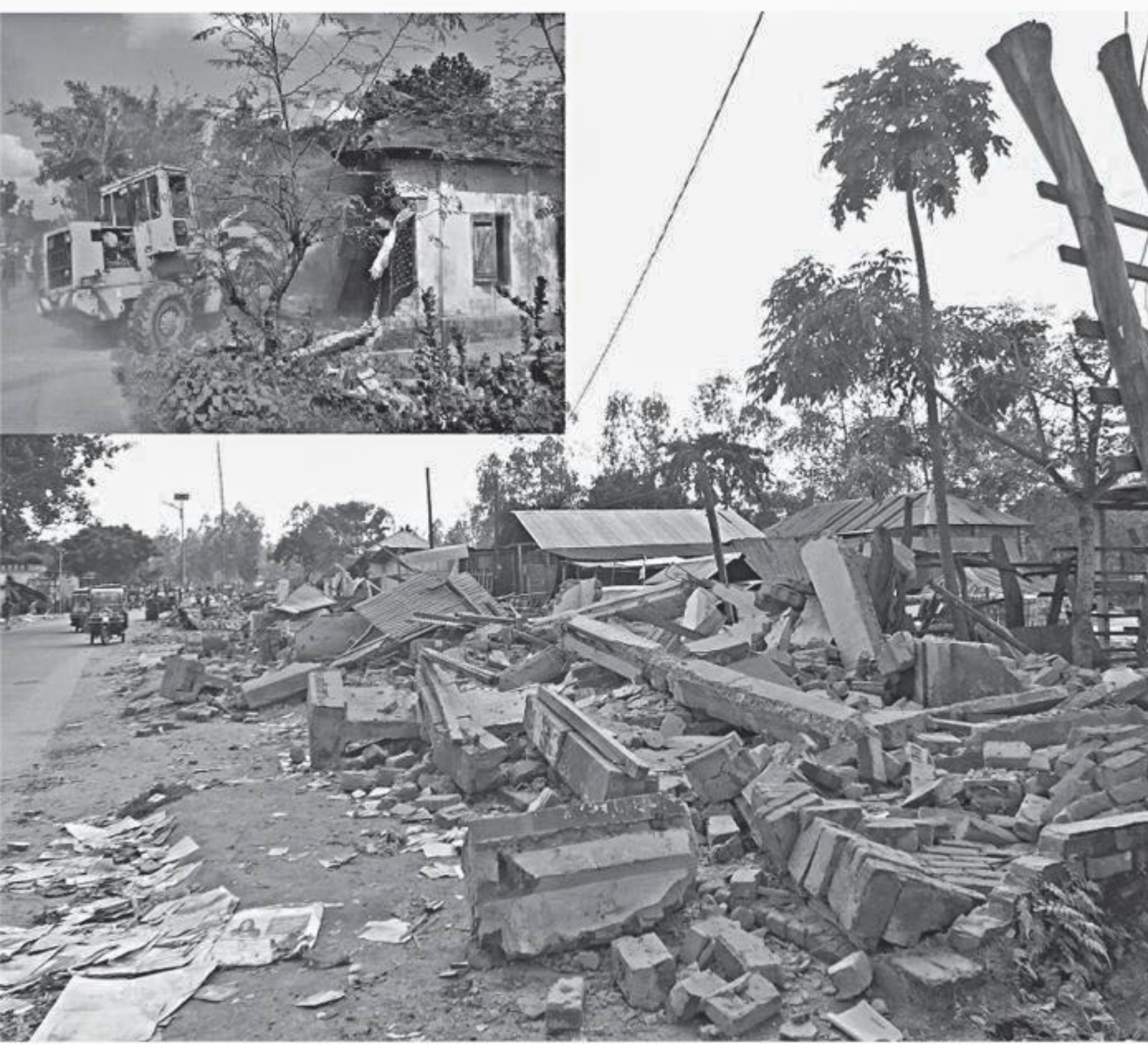
Nilphamari Roads and Highways Department (RHD) in an eviction drive on Saturday knocked down illegal structures beside Nilphamari-Domar regional highway in Sadar upazila.
