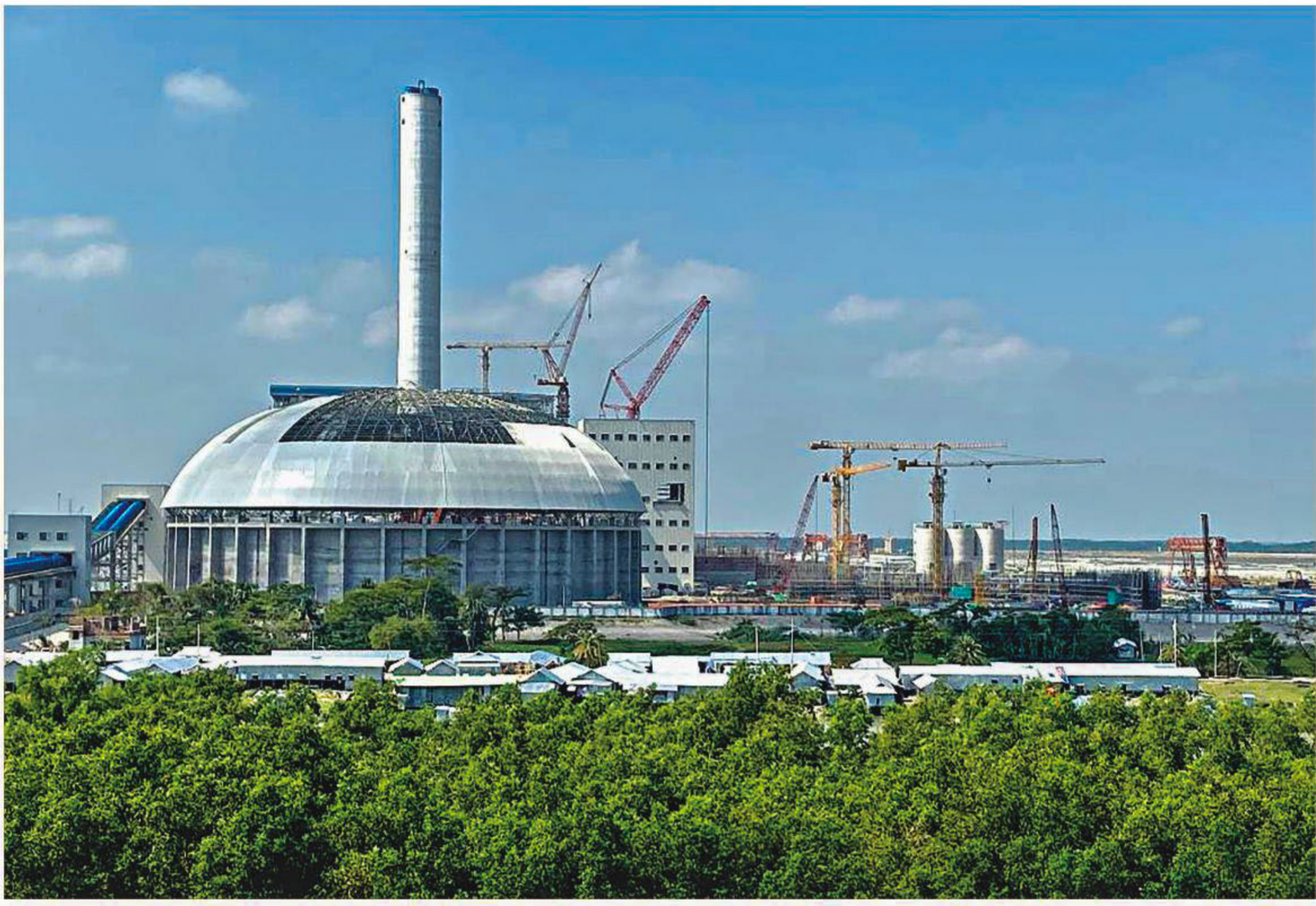
The coal storage silo of the under-construction 1,320MW Payra Power Plant in Patuakhali's Kalapara upazila. The plant's first unit, having a capacity of 660MW, is likely to be commissioned in January. The photo was taken on Tuesday.
