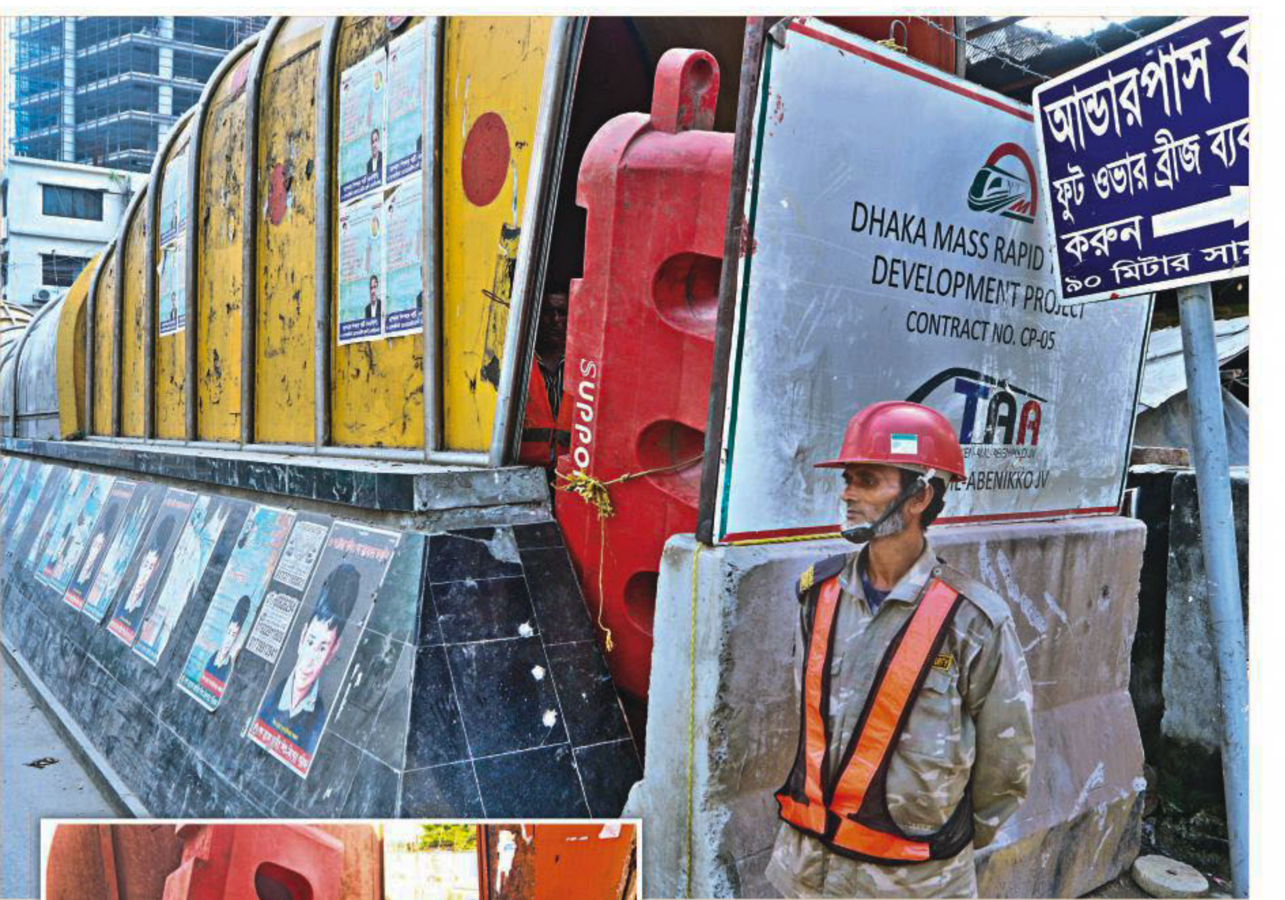
A guard standing by the sealed off entry to the underpass on Kazi Nazrul Islam Avenue at Karwan Bazar yesterday. The authorities appear to have tightened the measures after The Daily Star published a photo, inset, on Tuesday of people sneaking inside the underpass amid heavy construction work in the area. PHOTO: STAR
