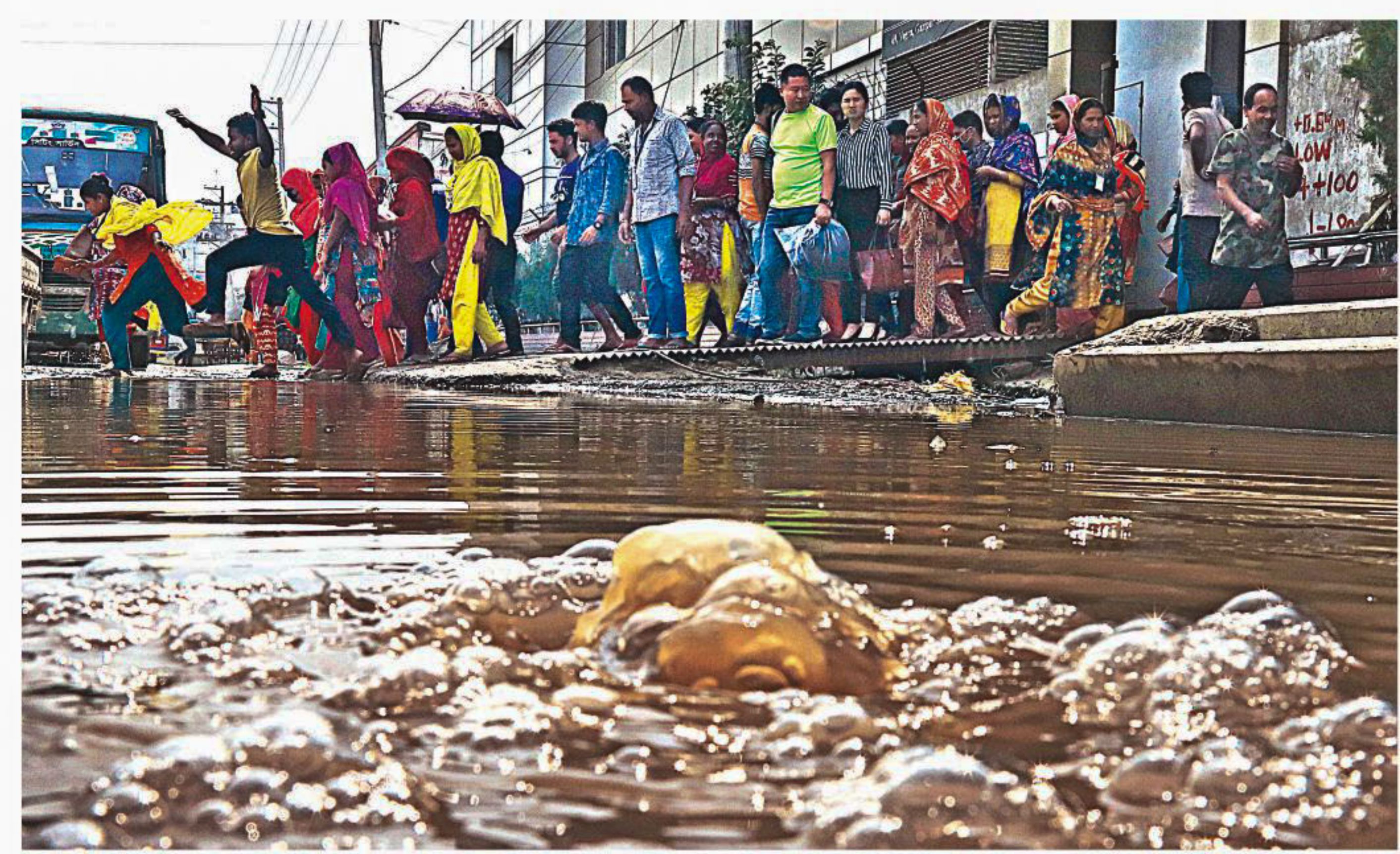
Pedestrians leaping over mud and water accumulated on roads is a common occurrence. Bubbling water, however, is not. Authorities had dug up this road, and in the process damaged a gas line underneath. The road was later patched up, but not the pipeline, said locals. Besides gas fuel being wasted, this could also turn into a fire hazard when the water recedes. The photo was taken on Tuesday from Maleker Bari area in Gazipur.
