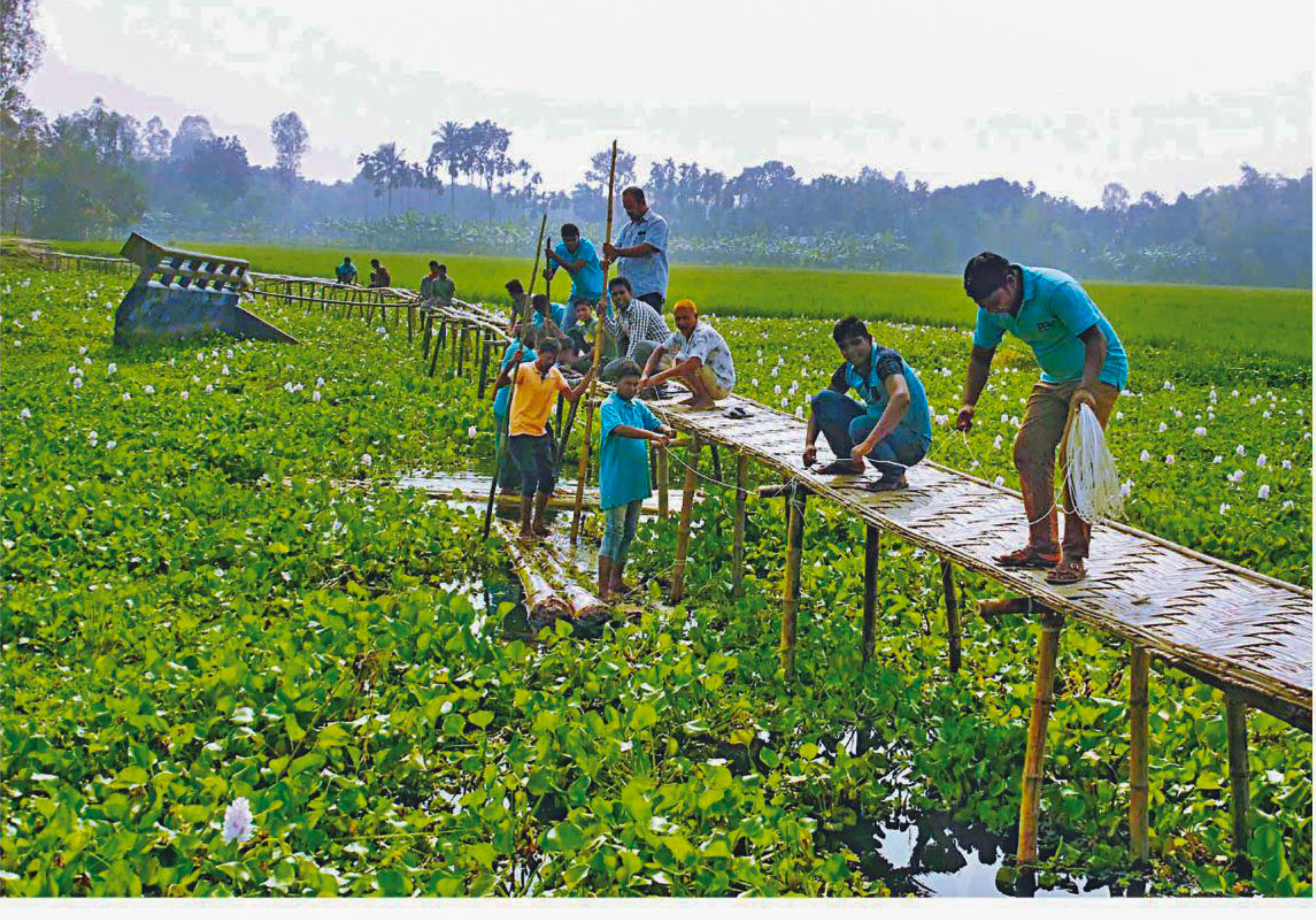
Locals building a bridge with bamboo on a canal in Gaddimari village of Lalmonirhat's Hatibandha upazila. They are putting in the effort after failing to get any help from the authorities to repair a bridge that collapsed in 2015. The photo was taken on Friday.
