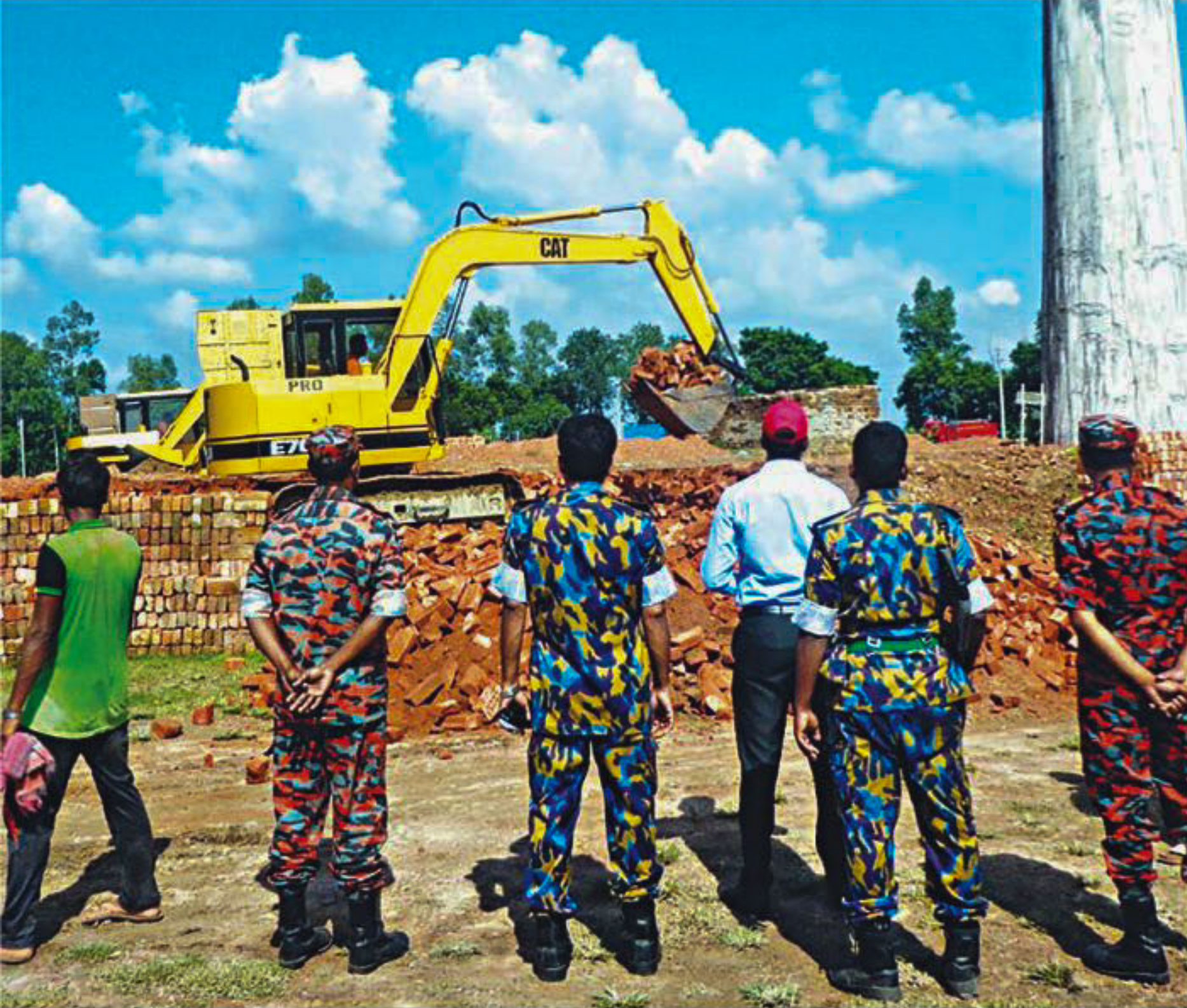
A mobile court during a drive yesterday demolished this brick kiln in Madla area under Bogura Sadar municipality.
