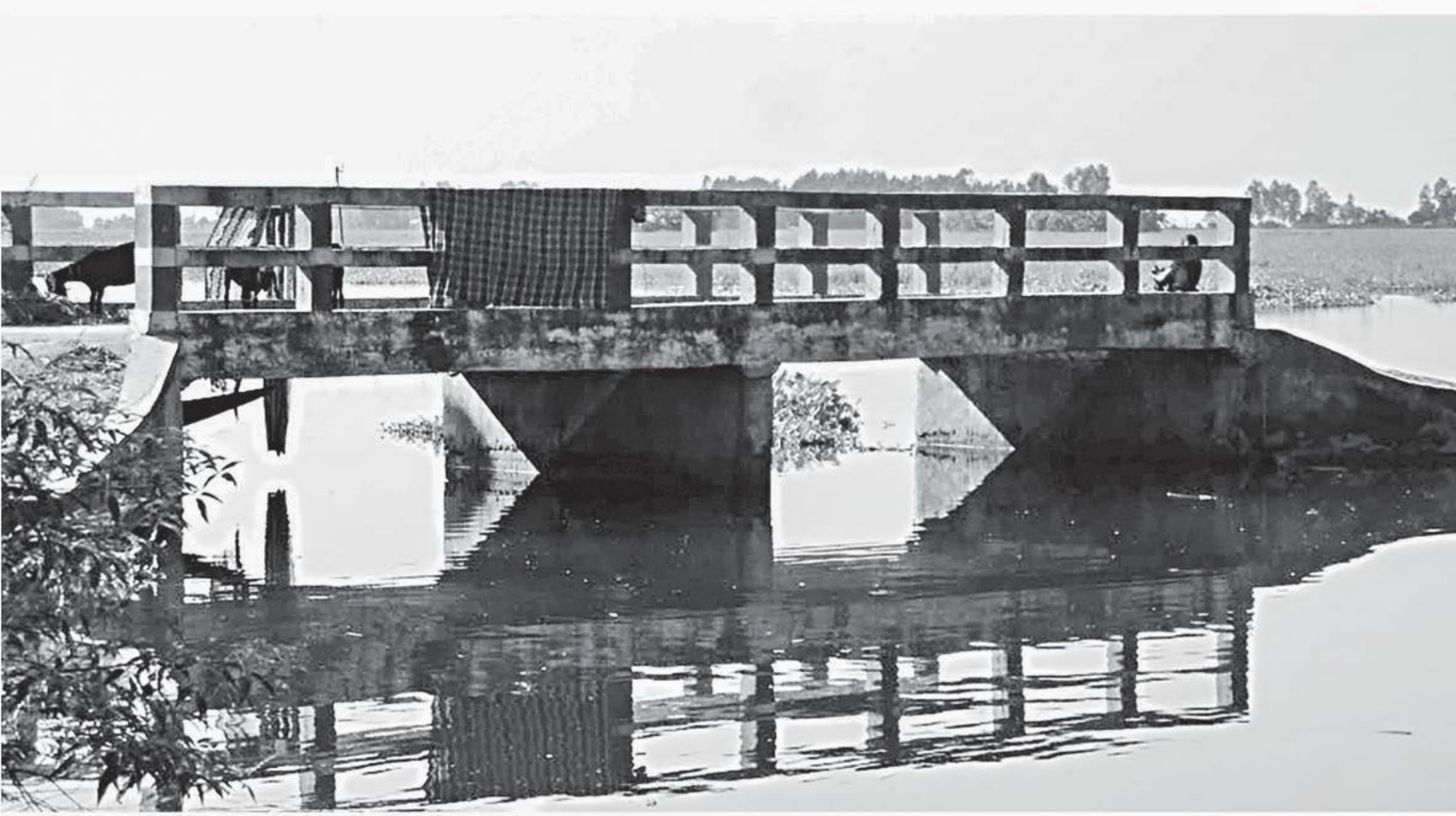
Built two years ago, this bridge over a canal at Shaguta village in Pabna's Sujanagar upazila is of no use to locals as there is no approach road on either side of the concrete structure.
