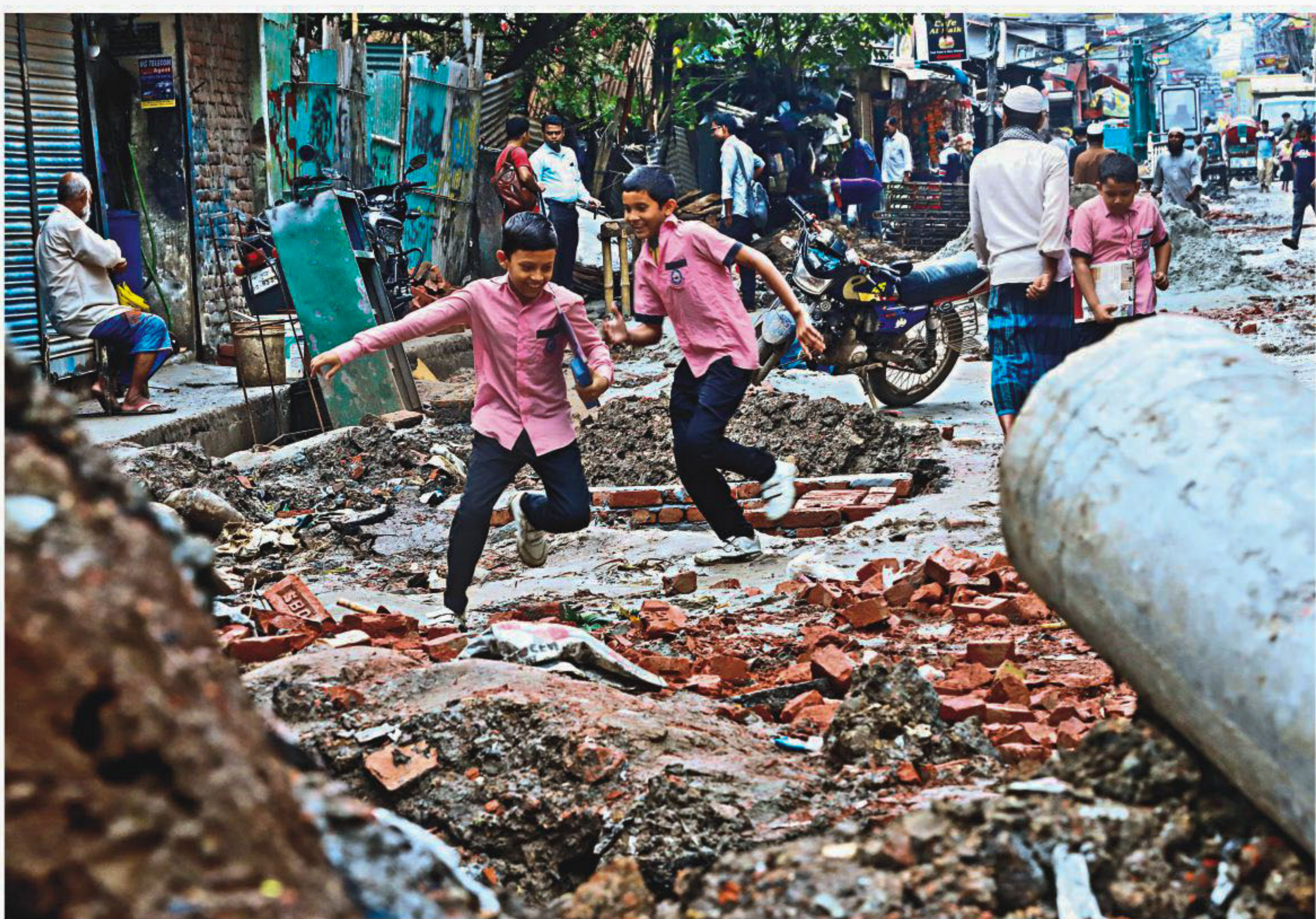
With construction materials lying haphazardly on the already dug-up road, walking on Mugda-Manik Nagar Wasa Road is no less than partaking in adventure sports. The road has been in this condition for over a month. These three friends were seen making the best of this frustrating situation on Saturday while returning from school.
