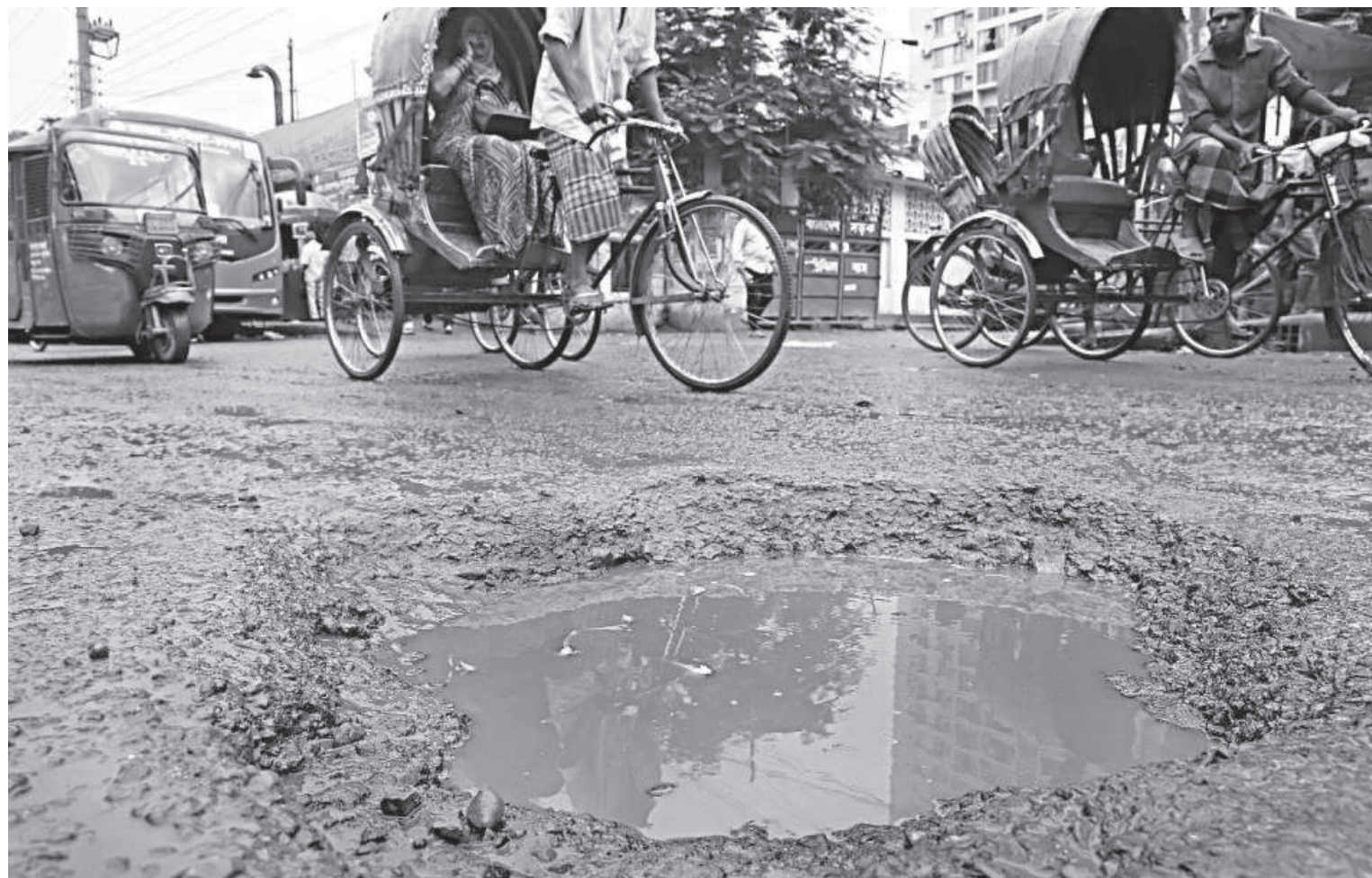
Large potholes at places and muddy surface have made travelling on this road in front of Kamalapur BRTC bus depot a risky and challenging task. Buses leaving or arriving at the depot are often seen facing difficulties negotiating this stretch. The situation worsens when it rains. The photo was taken yesterday.
