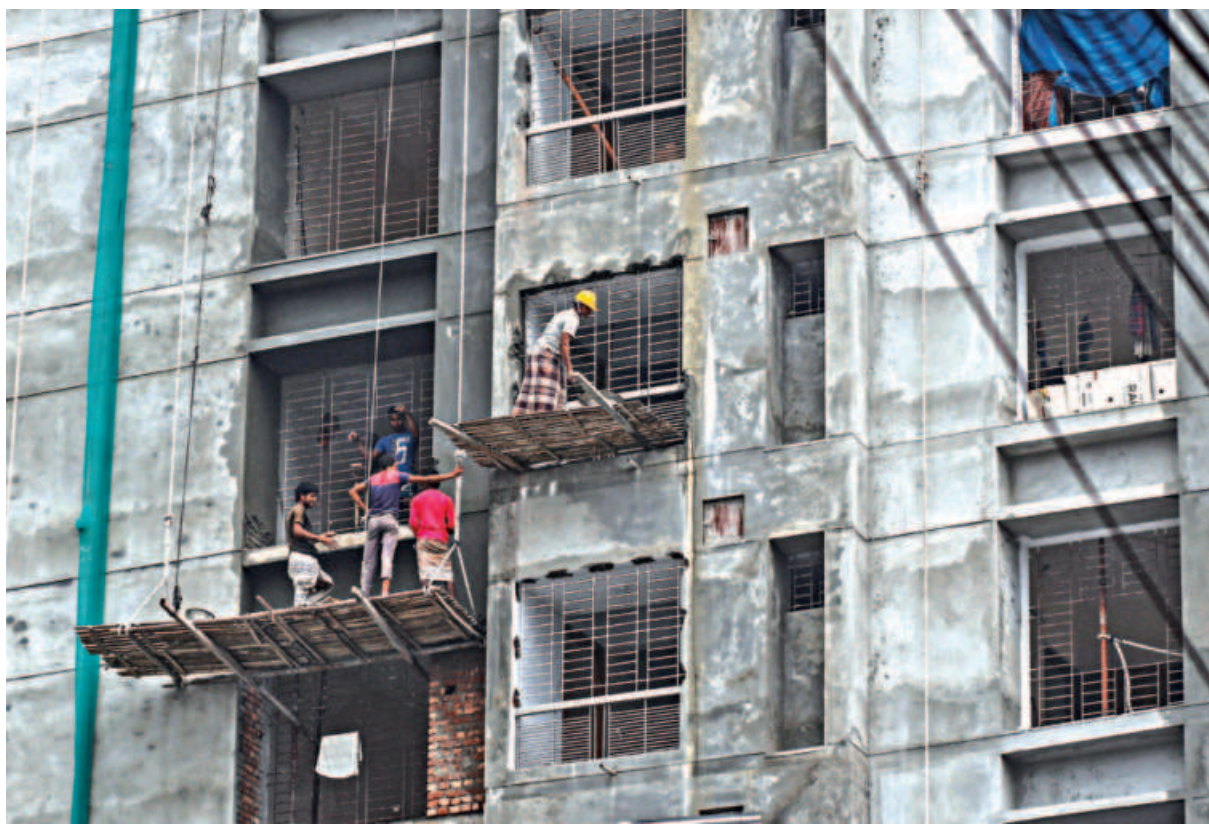
Workers hang off of the edge of a multi-storied building to complete the construction, in a highly unsafe working condition. The photo was taken recently from Dhaka's Nilkhet area.
