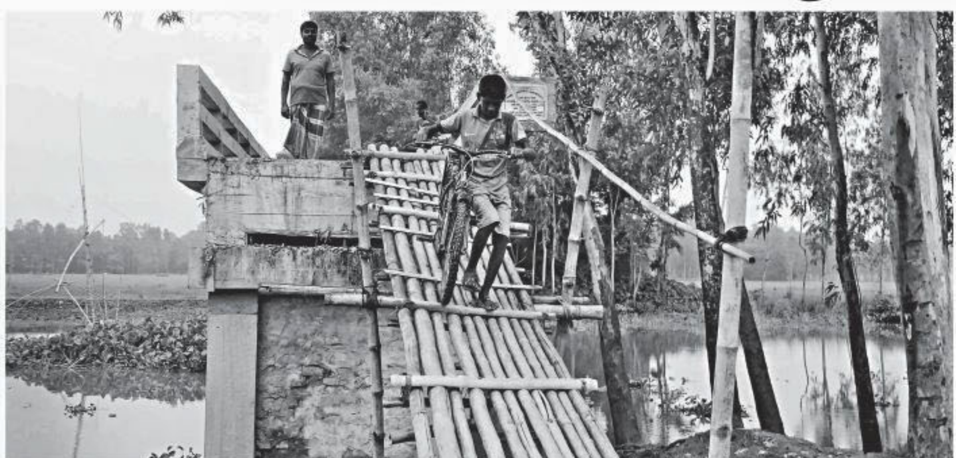
A bridge over a river causes immense sufferings to villagers in Tangail Sadar upazila as it does not have approach roads on either sides.
