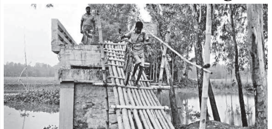
A bridge over a river causes immense sufferings to villagers in Tangail Sadar upazila as it does not have approach roads on either sides.
