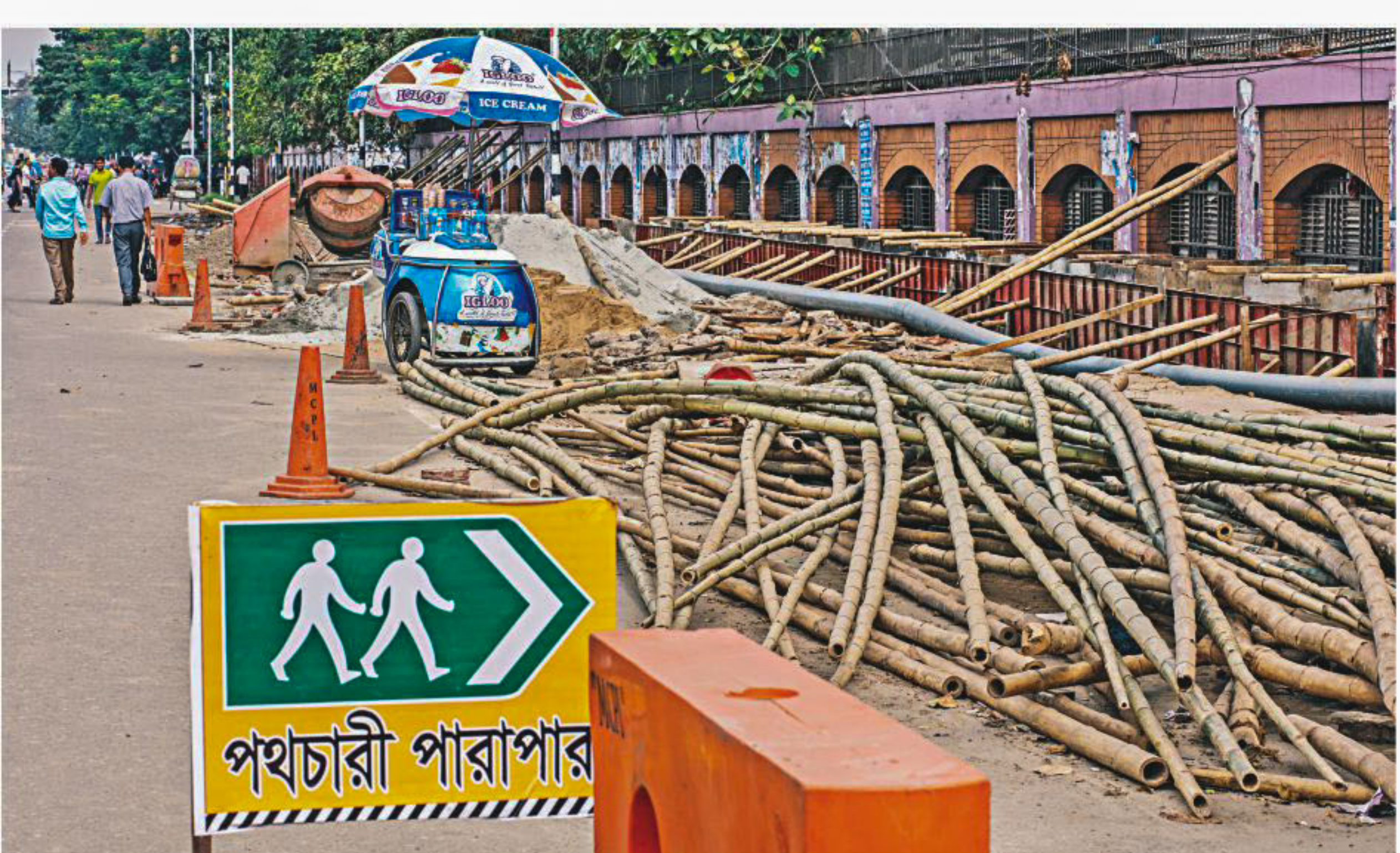
Drainage development works continue on Manik Mia Avenue, over a part of the footpath near Mirpur Road. Though the authorities concerned left some space beside the sidewalk for pedestrian movement along with a sign directing people to do so, it has been encroached by construction materials, a concrete mixture machine and an ice-cream van. The photo was taken recently.
