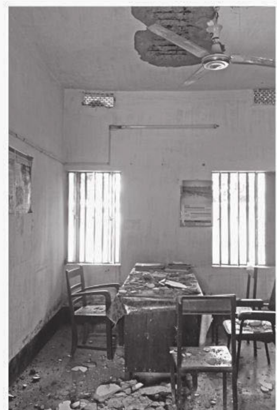
Heavy chunks of concrete fell from the ceiling in this room used by teachers at Madhabpur High School in Moulvibazar's Kamalganj upazila on Saturday evening.
