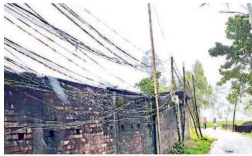
This cobweb of electric lines, held up by slanting bamboo poles in Pirjabad area of Rangpur town, can lead to accidents any moment. PHOTO: COLLECTED
