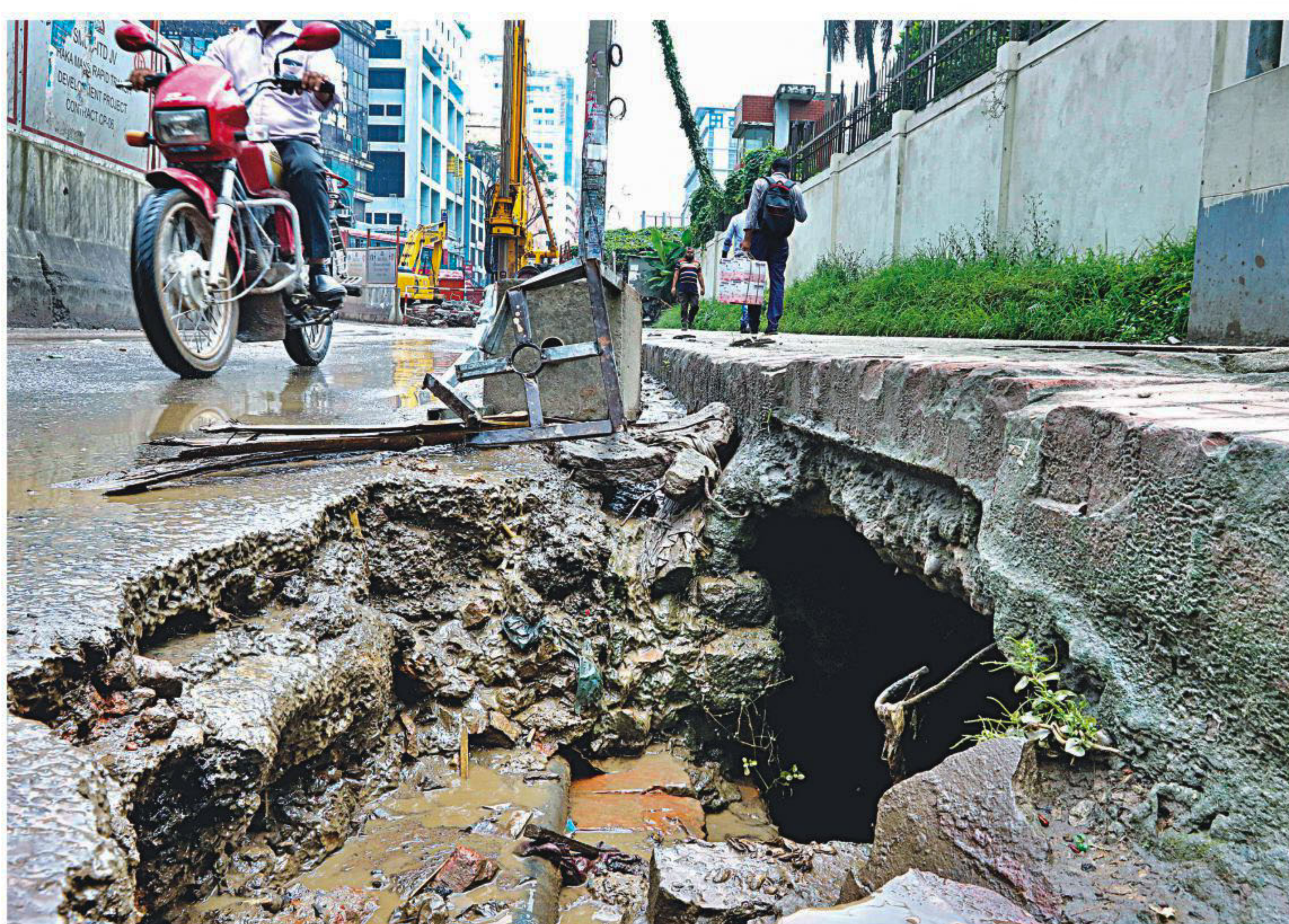
A huge crater along a footpath on Topkhana Road near the Secretariat in the capital. The road has been in this state for around two months, posing risks to both commuters and pedestrians.
