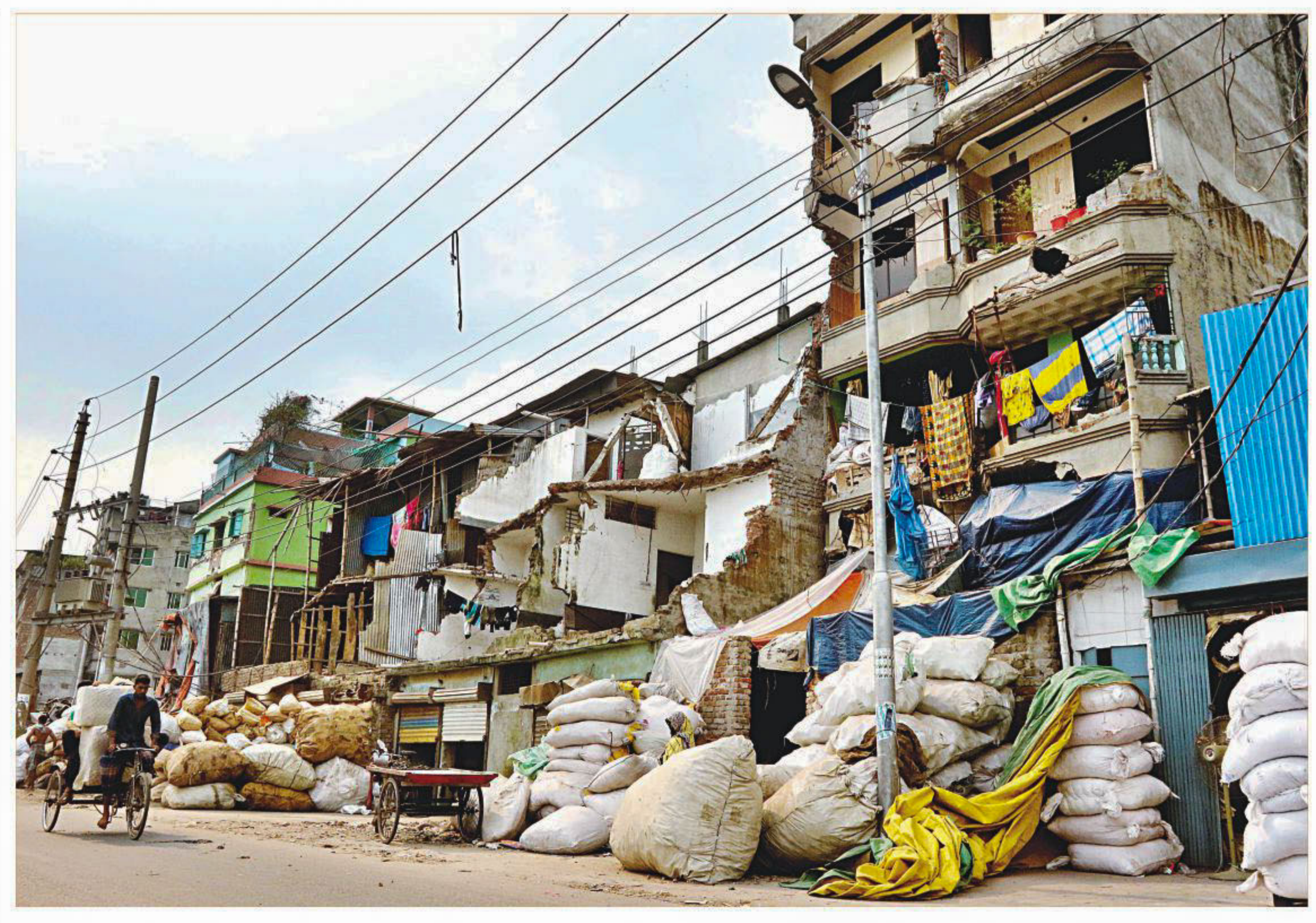
People are living in these partially-demolished buildings on Beribadh Road in the capital's Islambagh, putting their lives at risk. Parts of these houses along the Buriganga were knocked down by Bangladesh Inland Water Transport Authority during an eviction drive around eight months ago. The photo was taken earlier this week.
