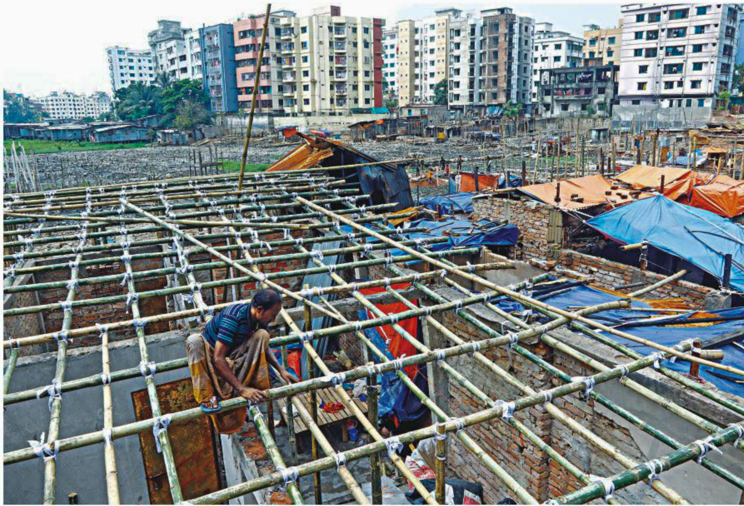
A man rebuilds a home which had burned down in fire at Mirpur's Chalantika slum in August. The photo was taken recently.
