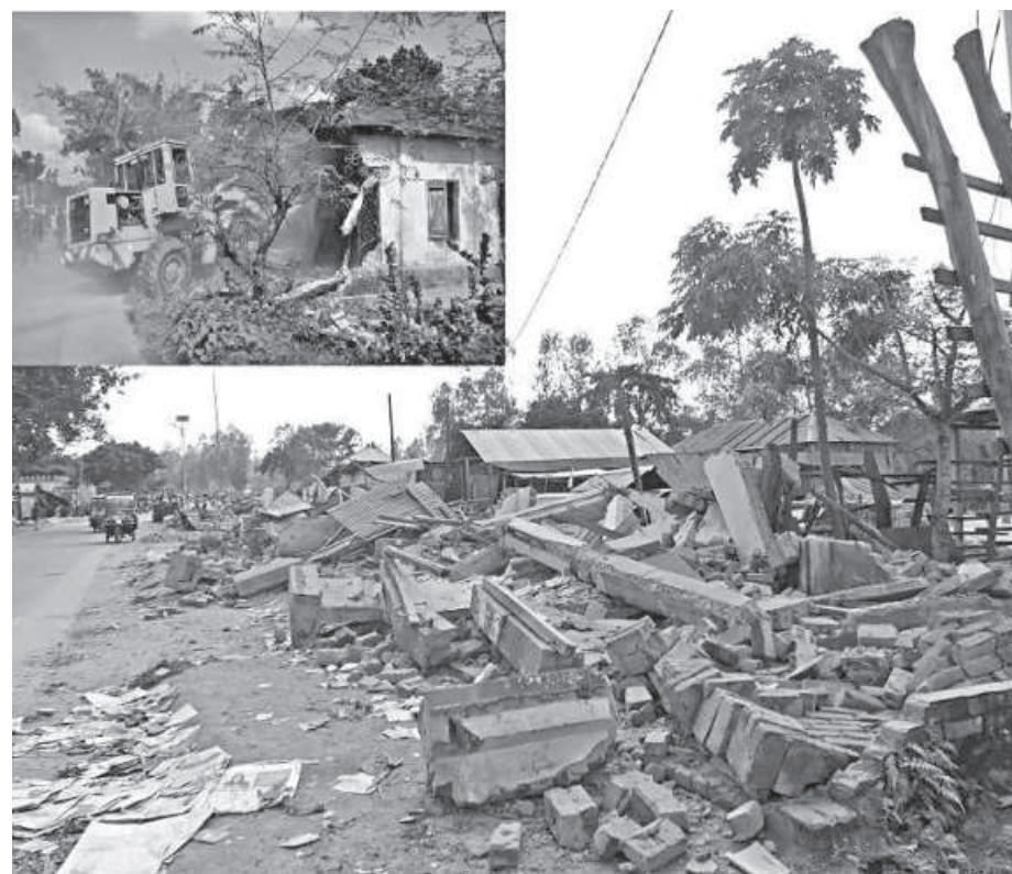
Nilphamari Roads and Highways Department (RHD) in an eviction drive on Saturday knocked down illegal structures beside Nilphamari-Domar regional highway in Sadar upazila.
