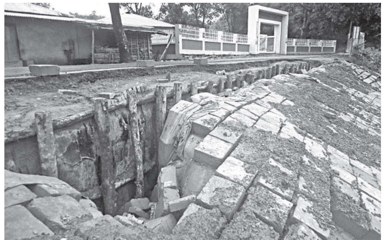
Amtali Para Government Primary School along with the neighbourhood remains in a vulnerable condition due to collapse of this embankment on the Sualok canal in Bandarban Sadar upazila.
