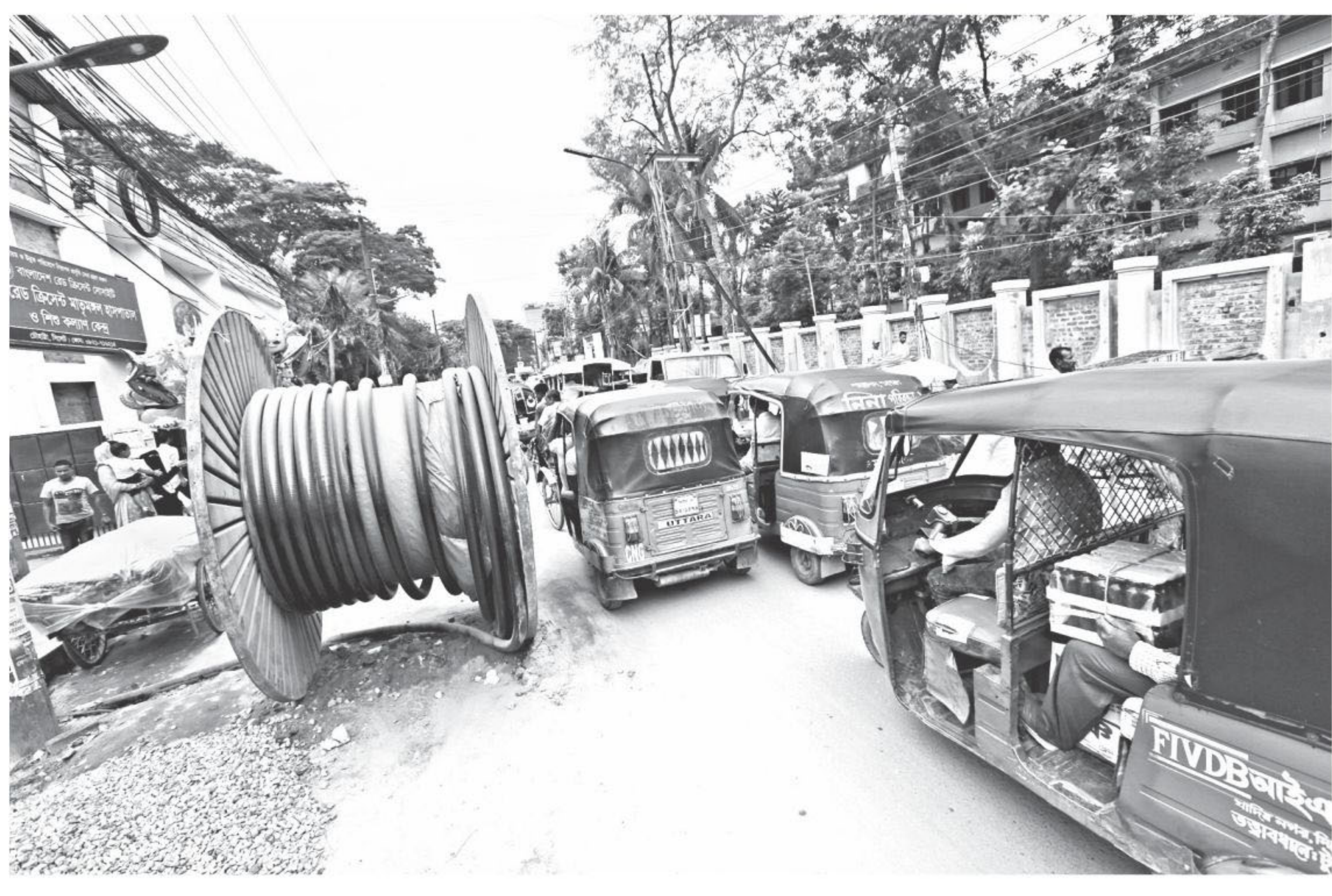
Vehicles are forced to move at a snail's pace on this part of a road in Sylhet city's Zindabazar area since a wooden cable reel and other construction materials have taken up almost half of its width. The authorities concerned have been working on Zindabazar-Chowhatta road for a long time to expand it and improve utilities. But due to the disorderly work, vehicles and pedestrians continue to bear the brunt. The photo was taken yesterday. PHOTO: SHEIKH NASIR
