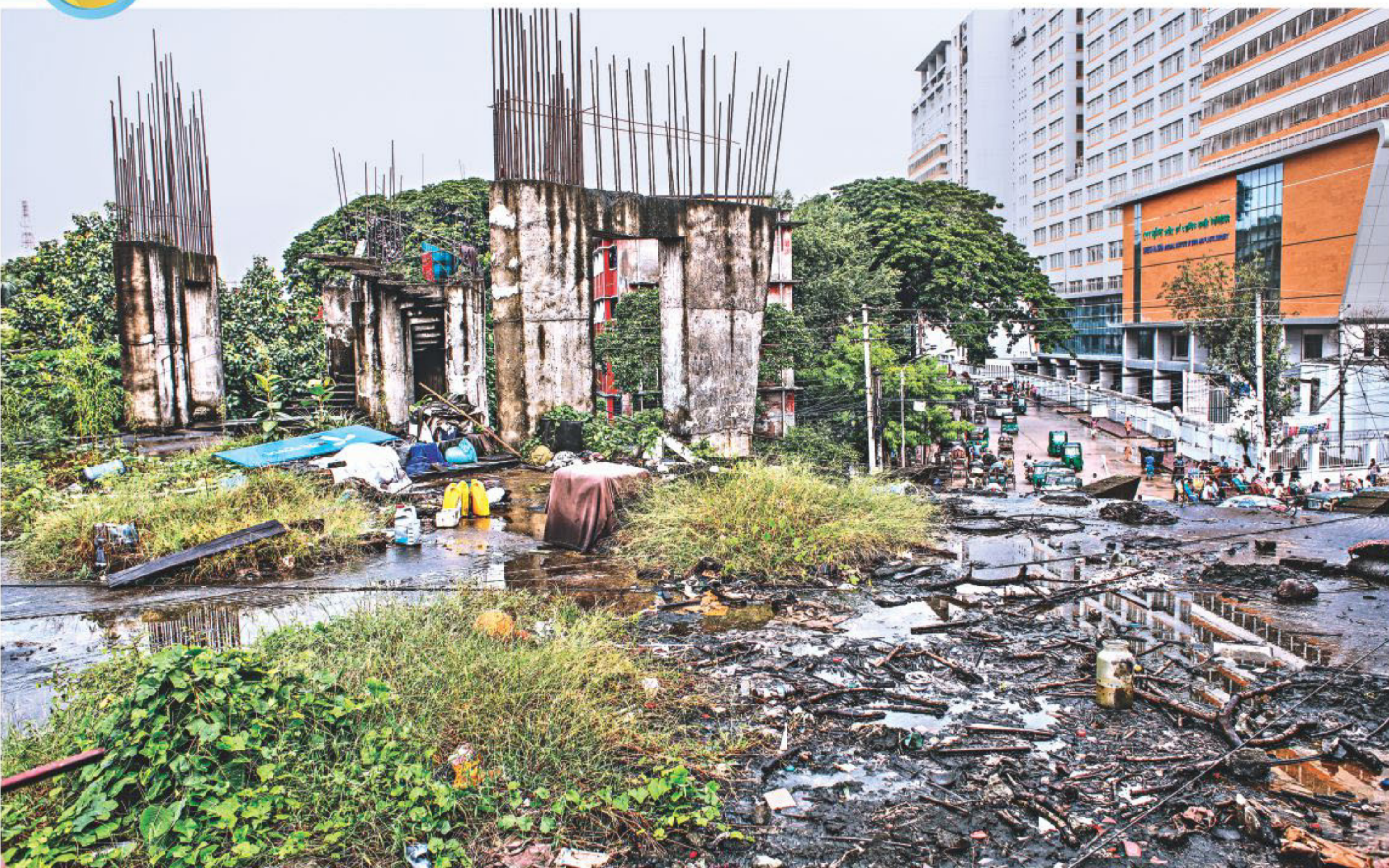
With iron rods poking out of concrete bases, this unfinished structure stands next to the historic Amtala site, where the Language Movement heroes defied Section 144 to demand Bangla as state language in 1952. Many of them embraced martyrdom in police firing. Work on this structure, near the emergency gate of Dhaka Medical College Hospital, started around a decade ago with an aim to construct a memorial in their honour. Now, not only does it remain forgotten, but is also surrounded by shrubs and garbage. The photo was taken yesterday.
