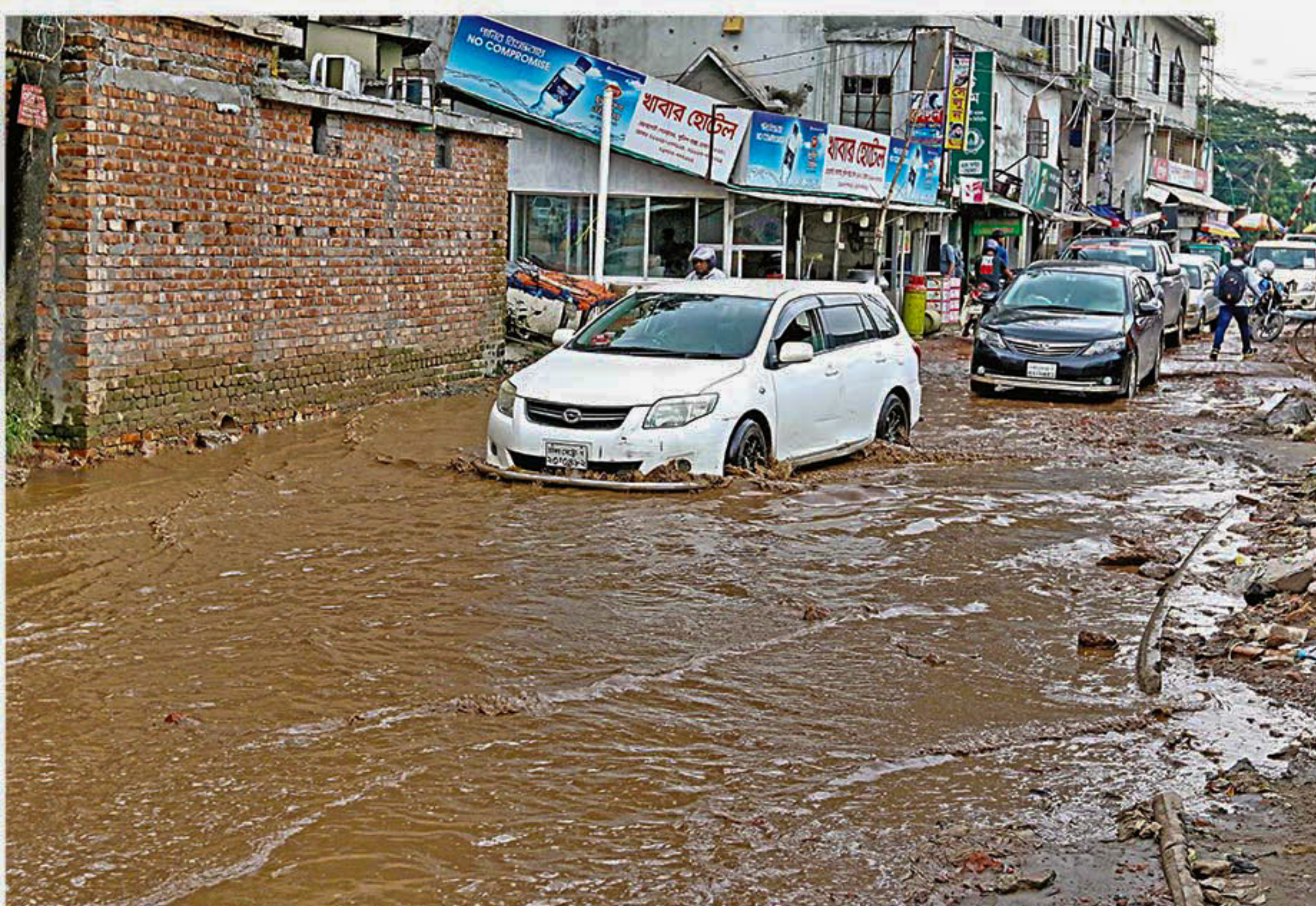
The road beside airport police box remains muddy and waterlogged due to lack of proper drainage system. Every day, vehicles heading towards the city from the airport use this alternate route as one side of the thoroughfare from Ashkona Hajj Camp to airport is closed to traffic because of the ongoing construction work of metro rail. The photo was taken yesterday.
