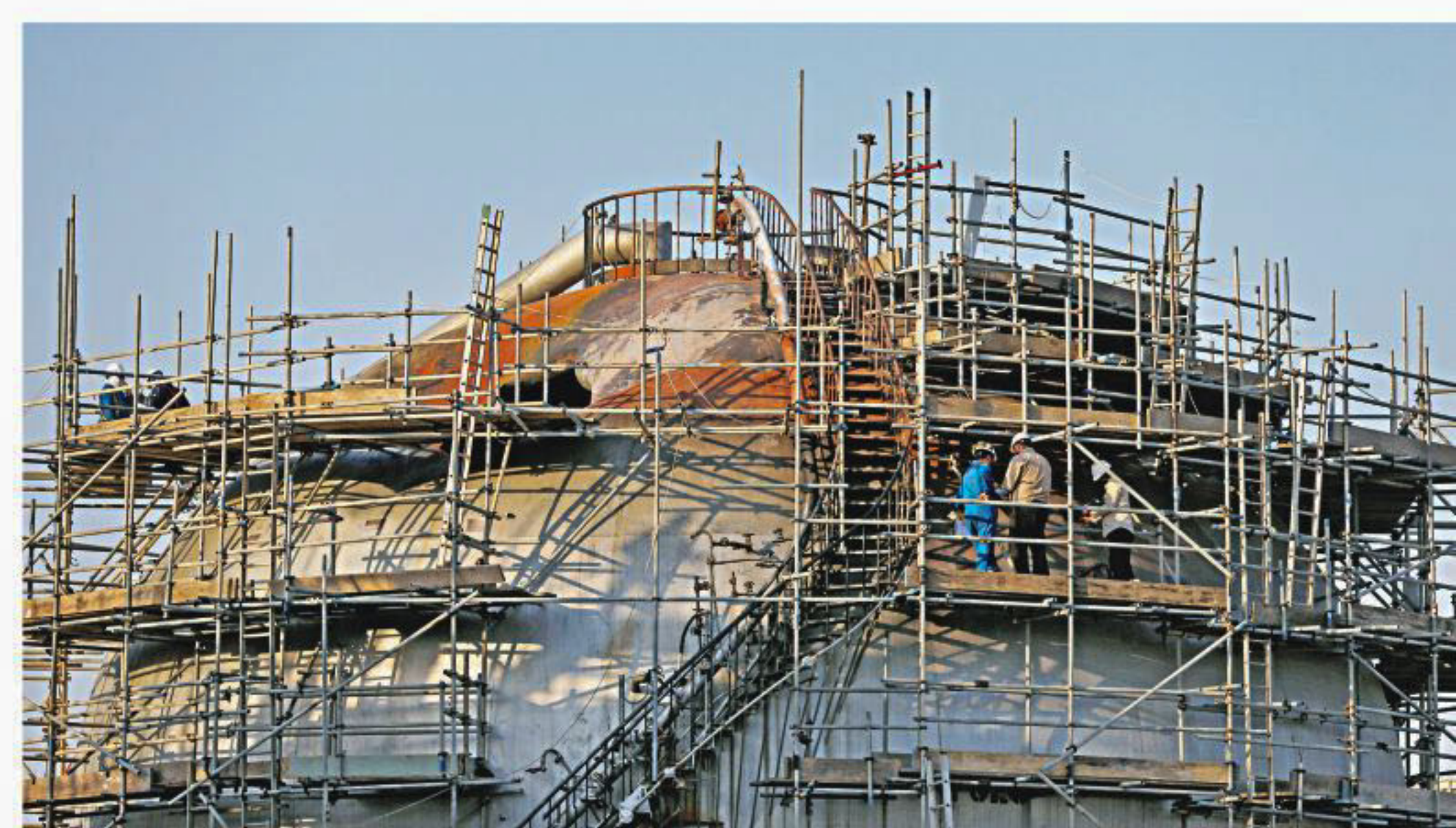
Workers are seen at the damaged site of Saudi Aramco oil facility in Abqaiq, Saudi Arabia.
