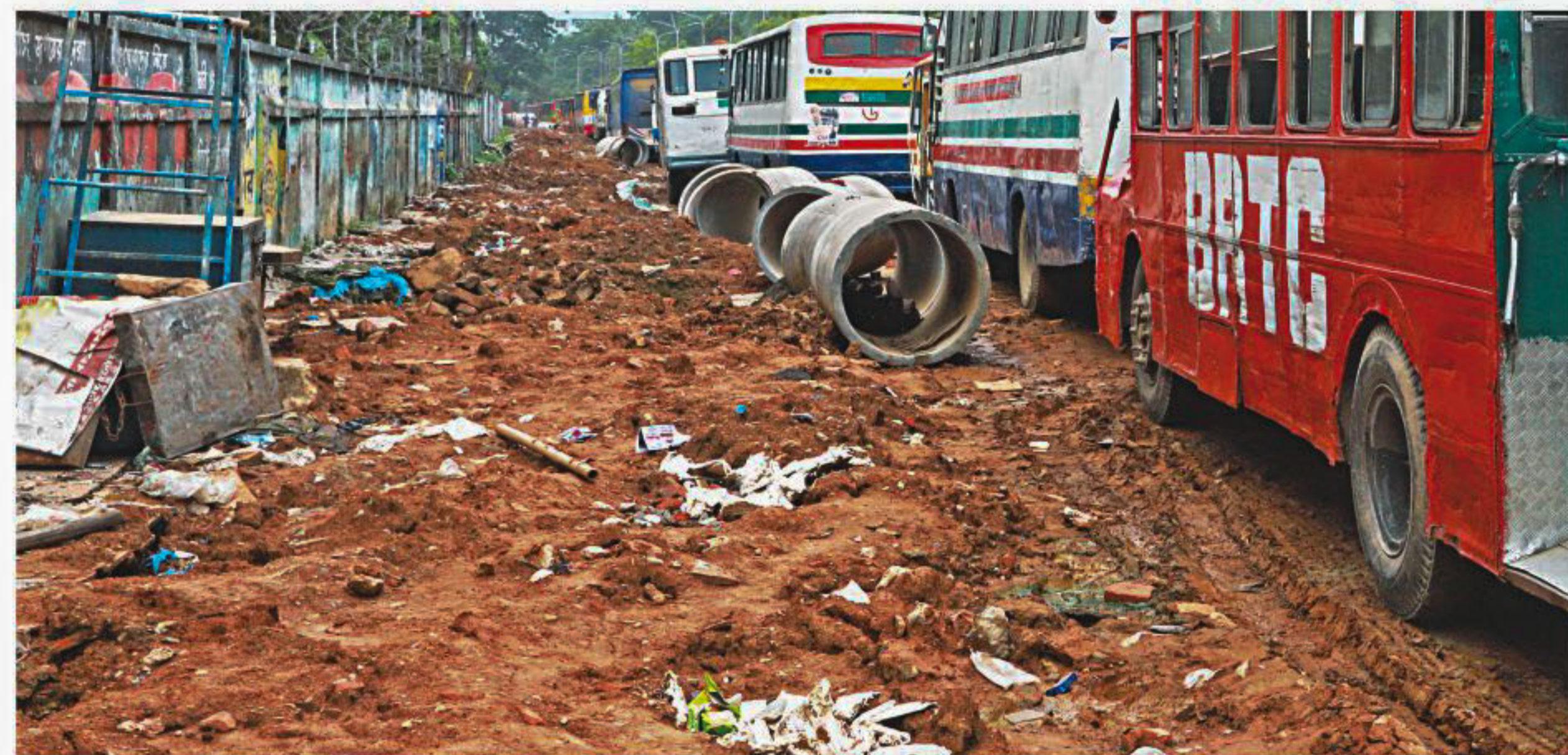
Sewerage pipes have been left on this road in the capital's Uttar Kamalapur for around two months, resulting in regular traffic congestion. Dhaka South City Corporation has been working on sewage line after digging up the road. The photo was taken yesterday.
