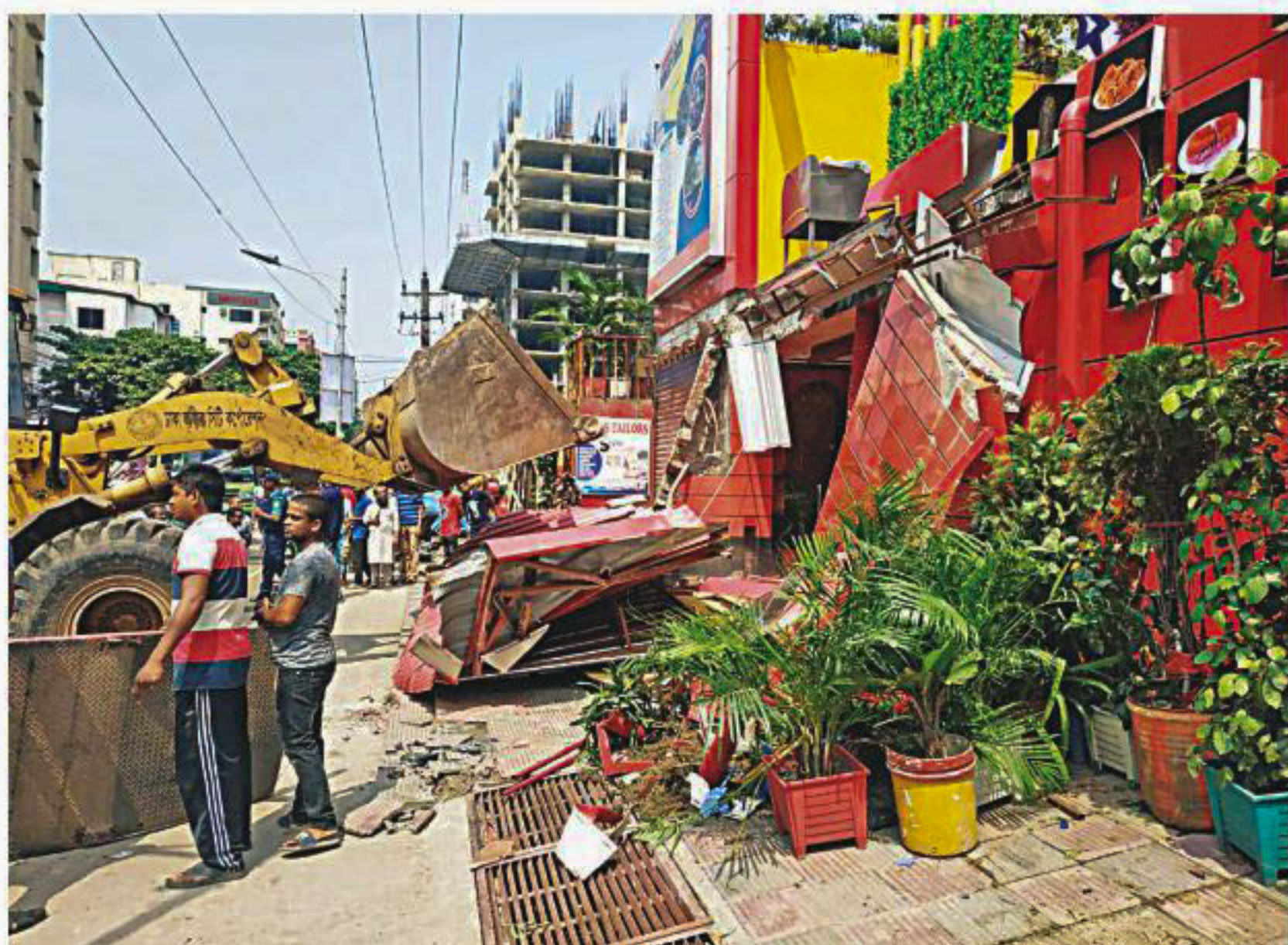
A DNCC excavator ploughs through a part of a restaurant that was extending on to the footpath near Garib-e-Nawaz area in Uttara. PHOTO: COLLECTED
