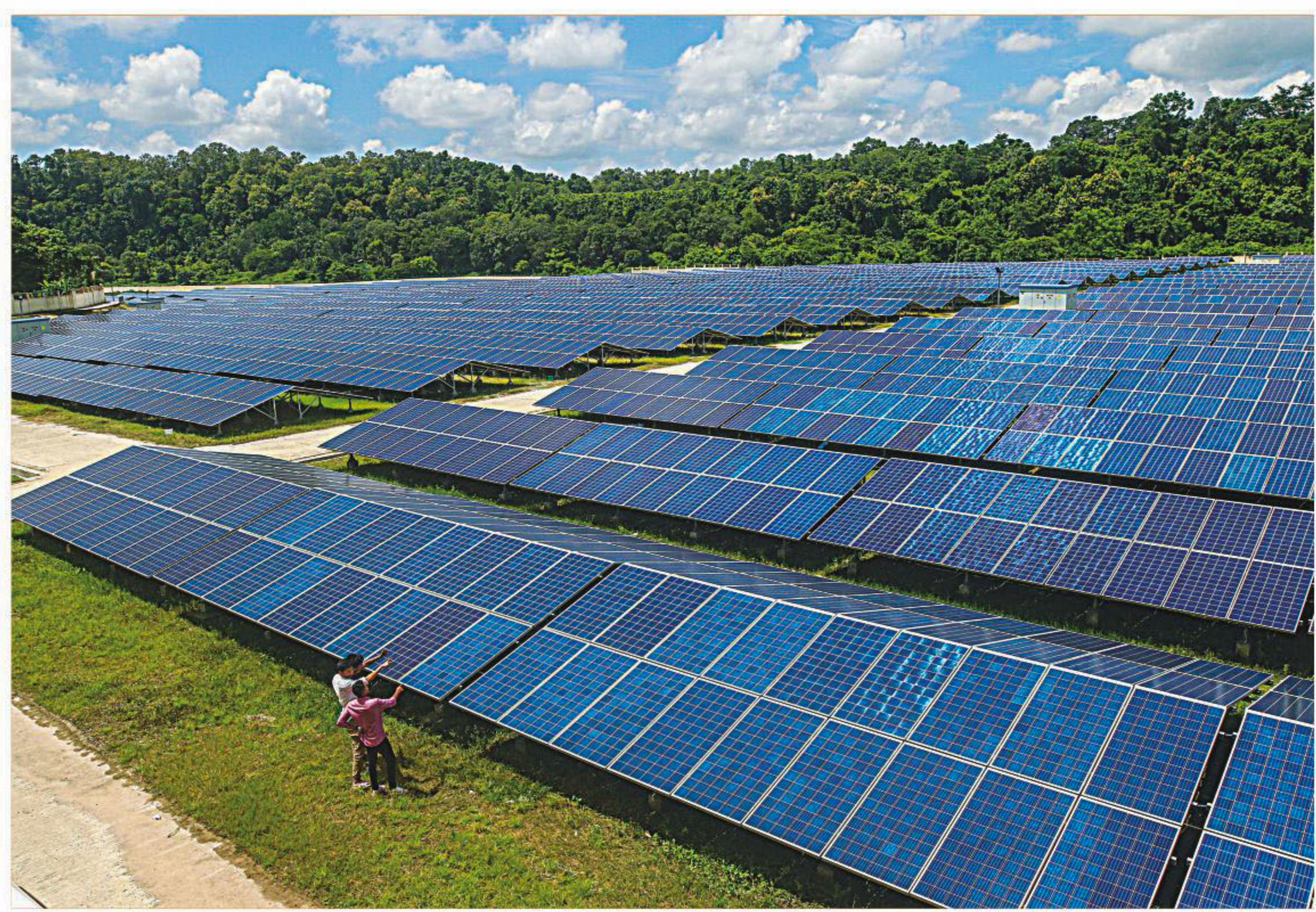
BYLINE: Solar panels set up near the Karnaphuli river as part of a power project in Rangamati. The project named "Kaptai 7.4-megawatt Solar PD Grid Connected Power Plant" was inaugurated by Prime Minister Sheikh Hasina on September 11. The picture was taken on September 16.
