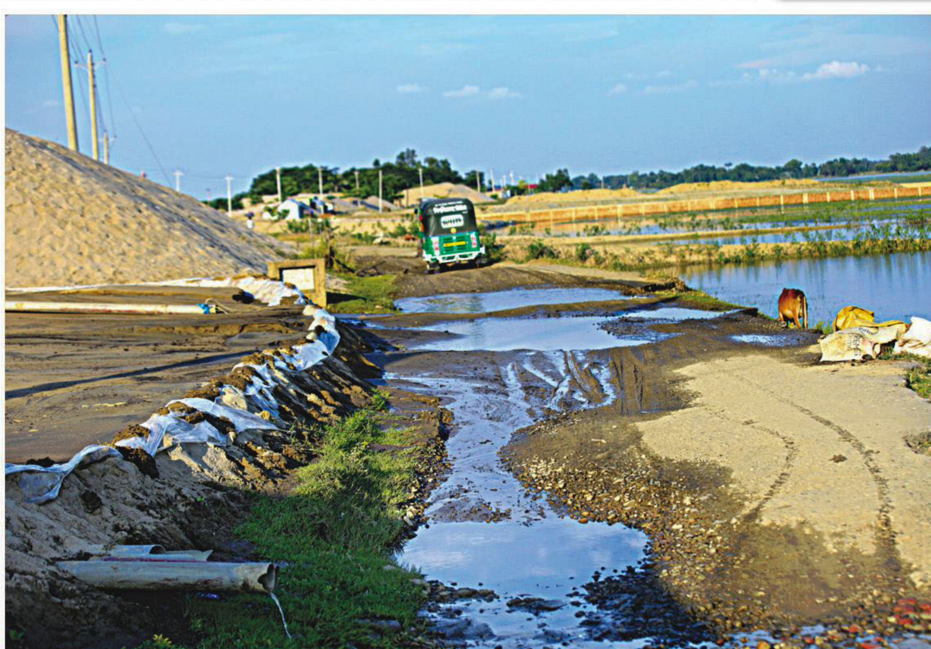
Loading and unloading of sand from trucks along the three-km-long Sylhet airport-Badaghat bypass road has left it riddled with potholes. Locals said the road is now almost inaccessible as some 40 traders sell sand in the area without caring much about the condition of the road. The photo was taken in Sylhet's Chamaurakandi area on Thursday.
