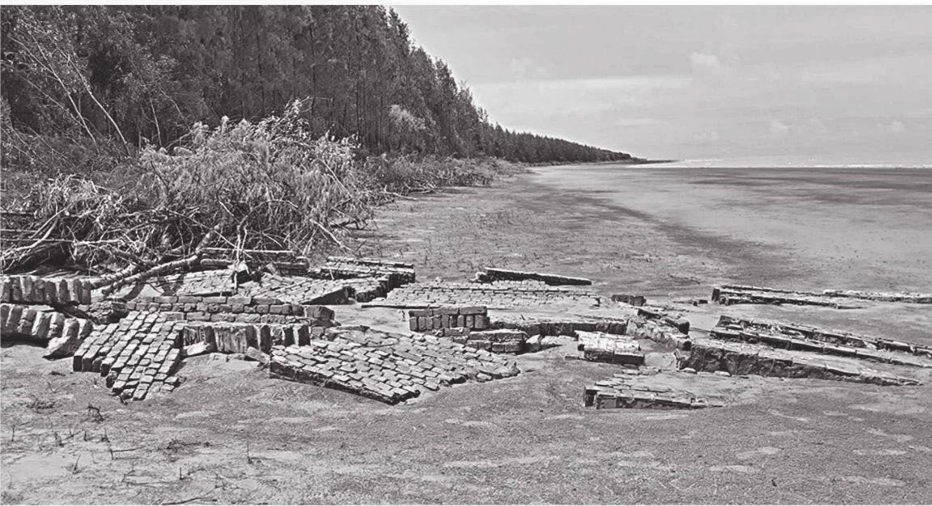
The damaged guide walls of link road between Barguna's Shubho Sandhya beach and Taltali town. The photo was taken recently.
