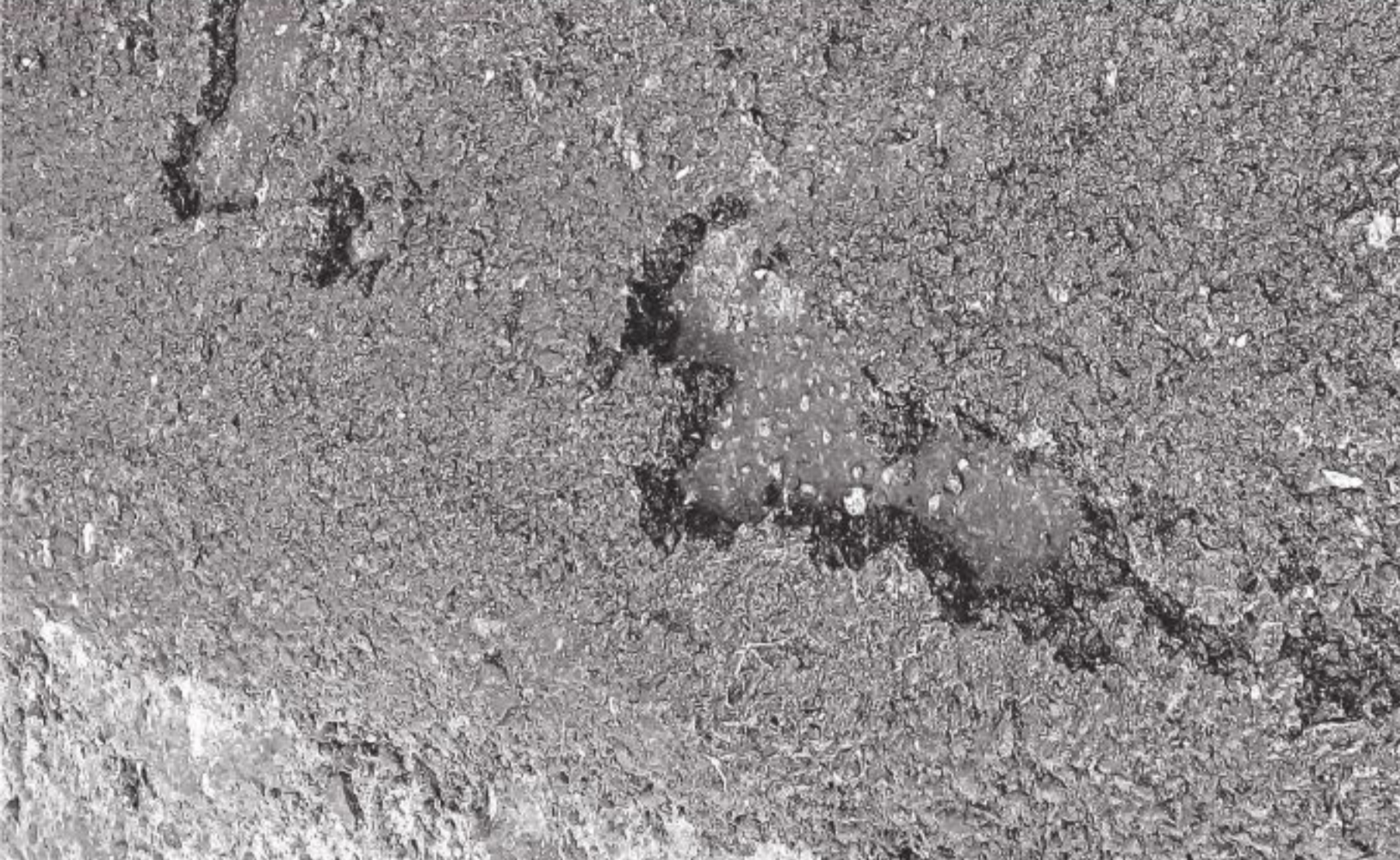
Two days after completion of renovation work of a five-km-long portion of Kulaura-Chandagram regional highway in Moulvibazar's Barlekha upazila, it gets damaged.
