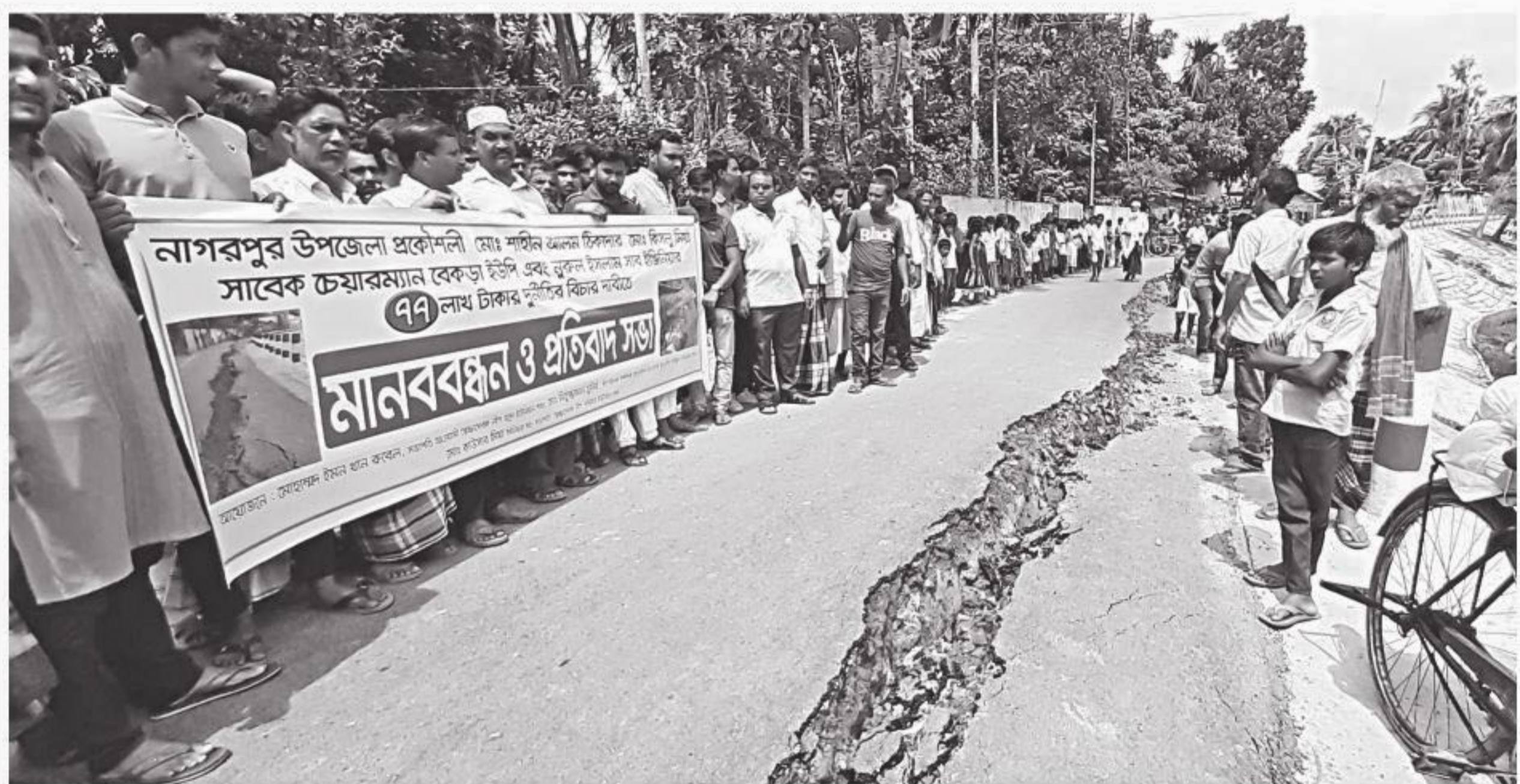
Hundreds of locals formed a human chain at Dhunail in Tangail's Nagarpur upazila last week, demanding action against the contractor concerned for using substandard materials in newly renovated Bhadra-Boptior road and the upazila engineer for his alleged negligence in supervising the road repair work.
