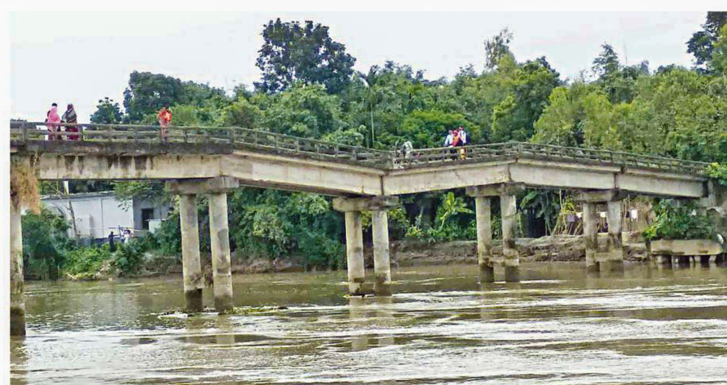
With pillars subsided in the middle, this awfully risky bridge on the Jhinai river at Dapnajor in Tangail's Basail upazila remains the lone means for people of several villages who have to cross the river for going to different places including district headquarters.
