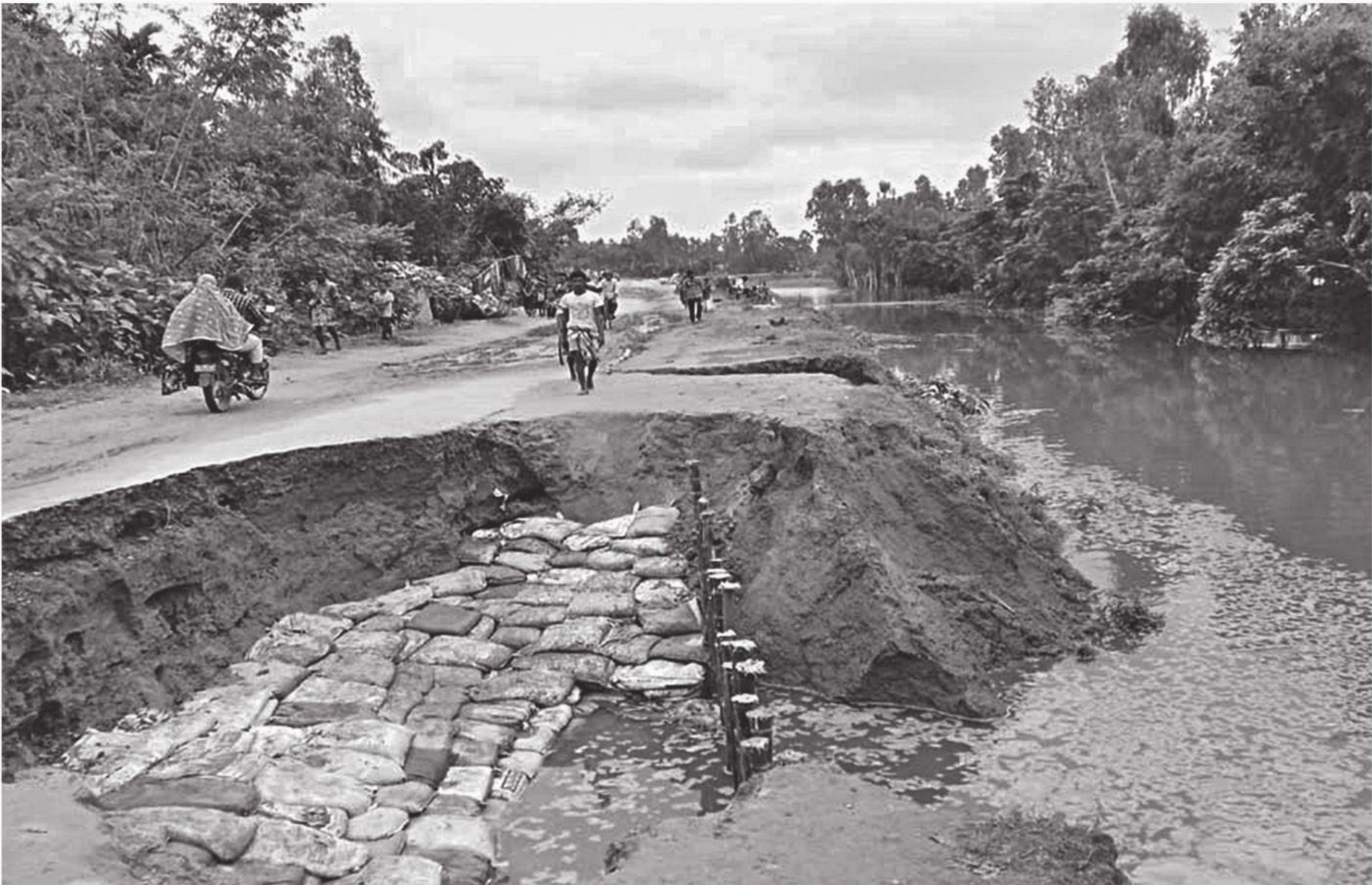
Like many other infrastructures damaged by the recent floods in Sundarganj upazila of Gaibandha, Belka-Sundarganj road cum flood control embankment remains without any repair.
