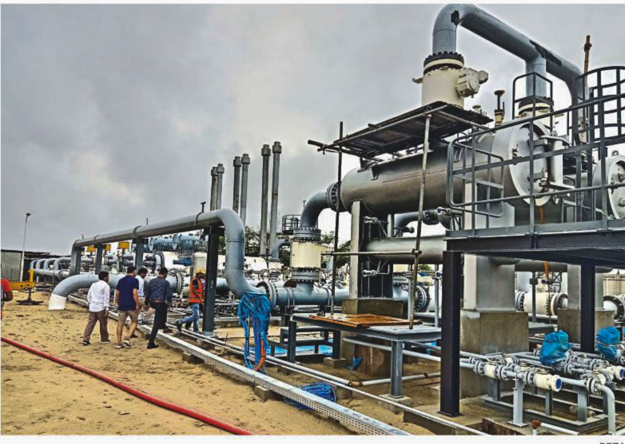
The photo shows a section of the gas supply facilities erected for industrial units inside Mirsarai economic zone.
