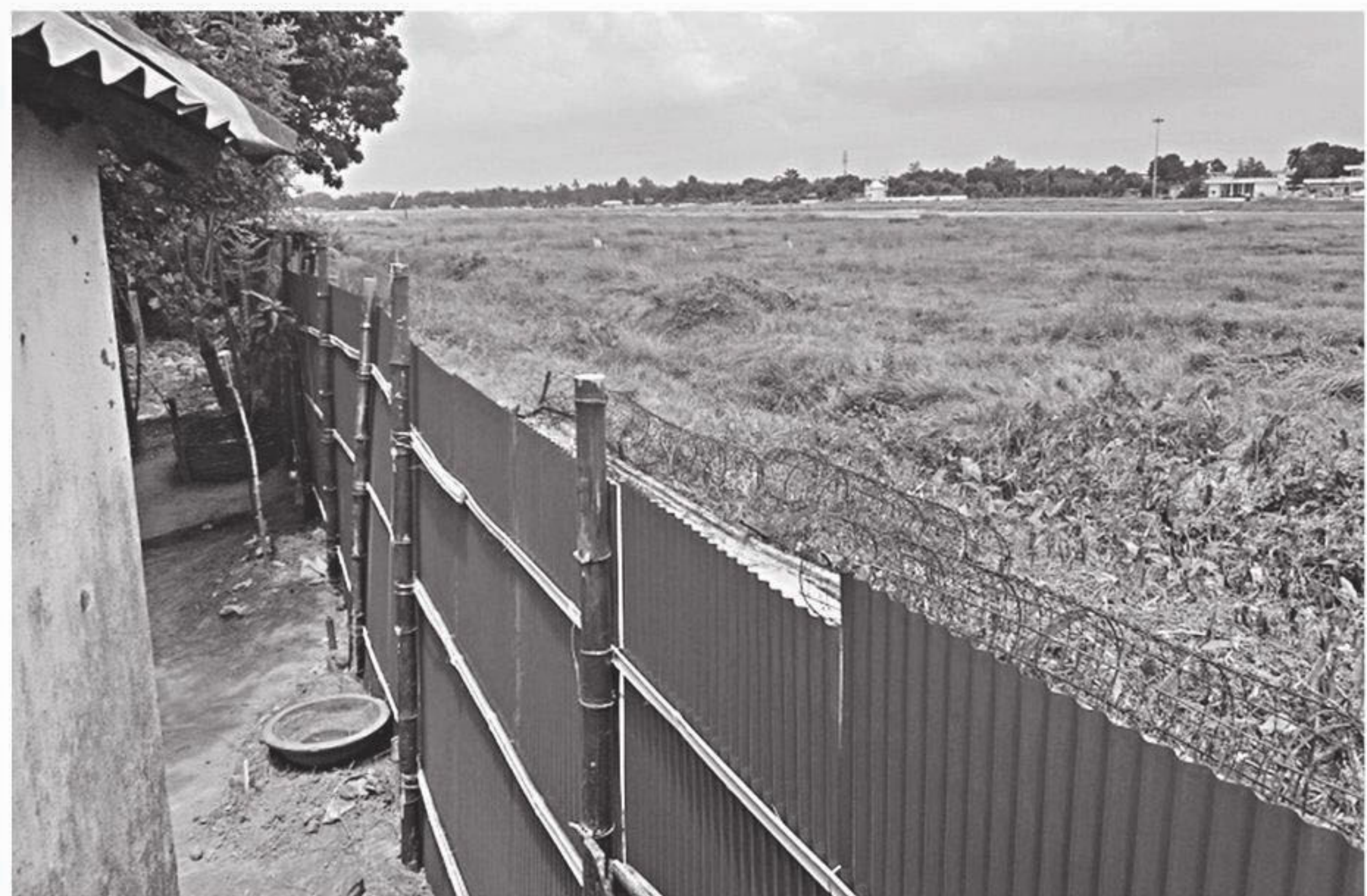
A makeshift fence with corrugated iron sheets and bamboo was made on Tuesday after a 60-foot stretch of boundary wall along the western side of Saidpur airport in Nilphamari collapsed on August 25. The security of the airport is now under threat and the authorities will have to spend more money to reconstruct the wall as the remainder of the wall has also tilted. Locals alleged that substandard material was used when the wall was built five to six years ago. PHOTO: EAM ASADUZZAMAN
