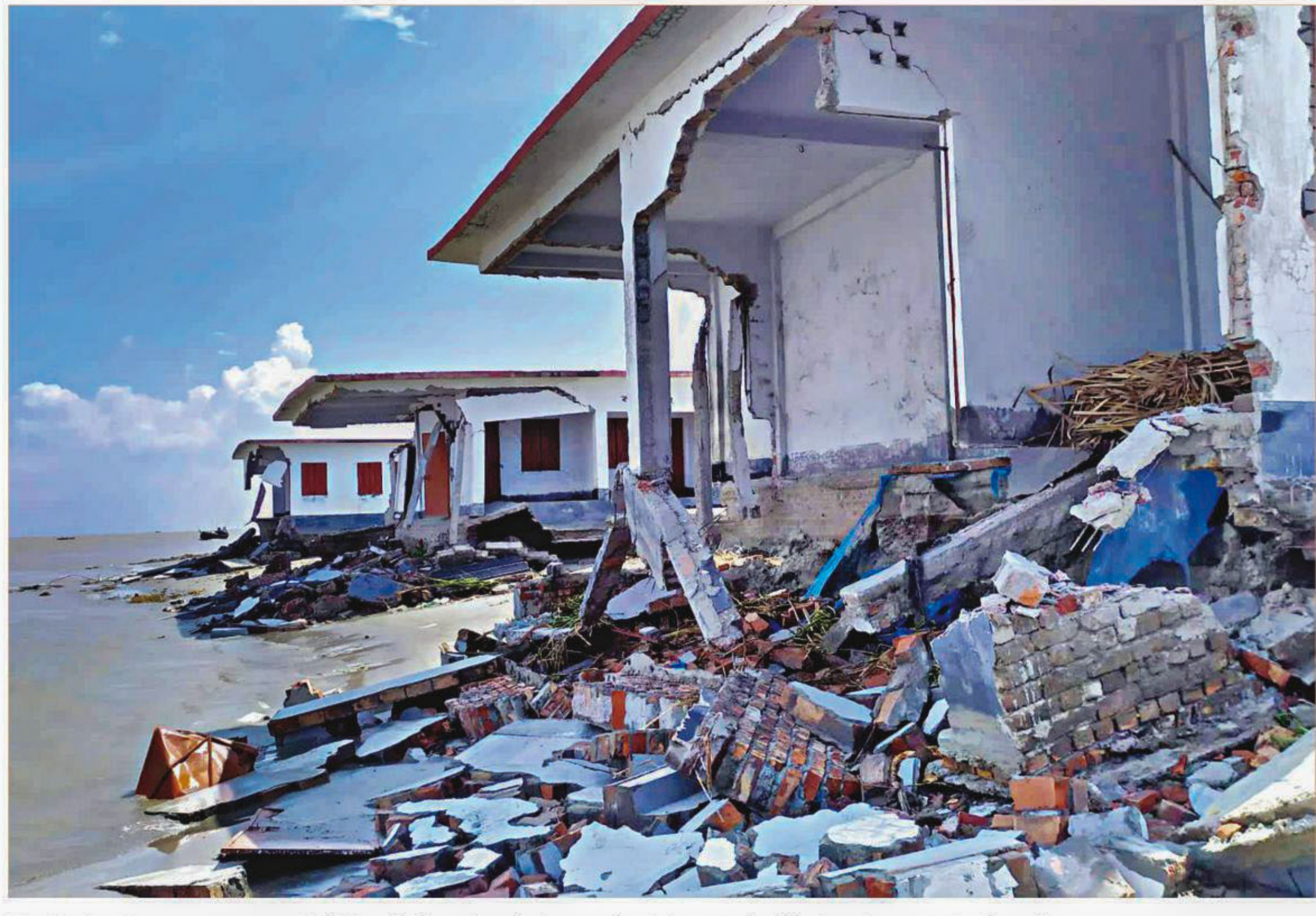
The Meghna lays waste to some buildings in Chandpur Sadar upazila. At least 25 families lost homes to the fury of the mighty river in the last seven days. The photo was taken a couple of days ago.
