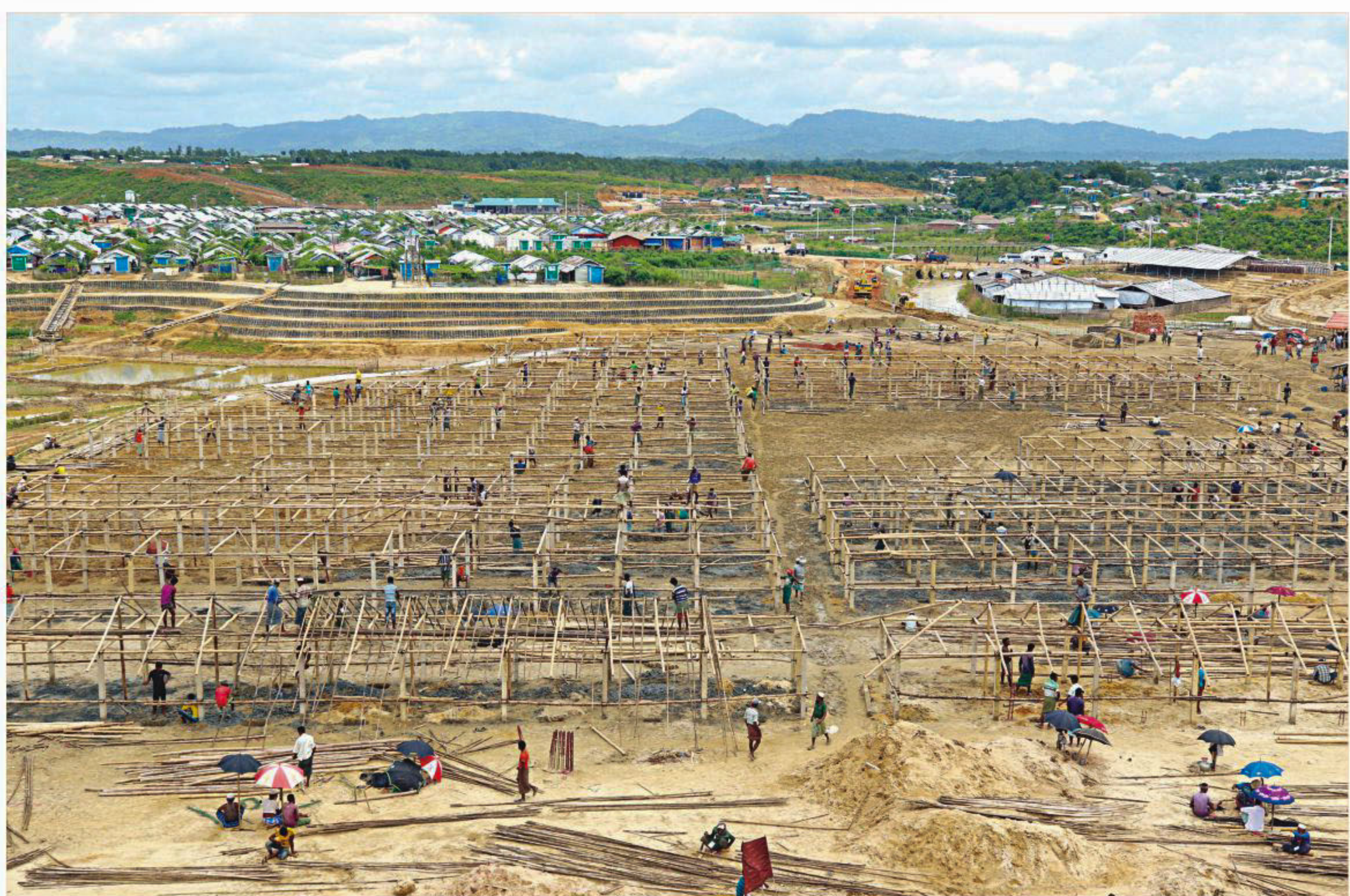
New settlements are being set up for Rohingya refugees at a field adjacent to the Camp-4 extension in Kutupalong of Cox's Bazar yesterday. A man, who was looking after the construction work, said the new houses were being built to give the refugees better living conditions. Only three days ago, thousands of Rohingyas staged a rally at this field, demanding justice for the atrocities the Myanmar military committed against them.
