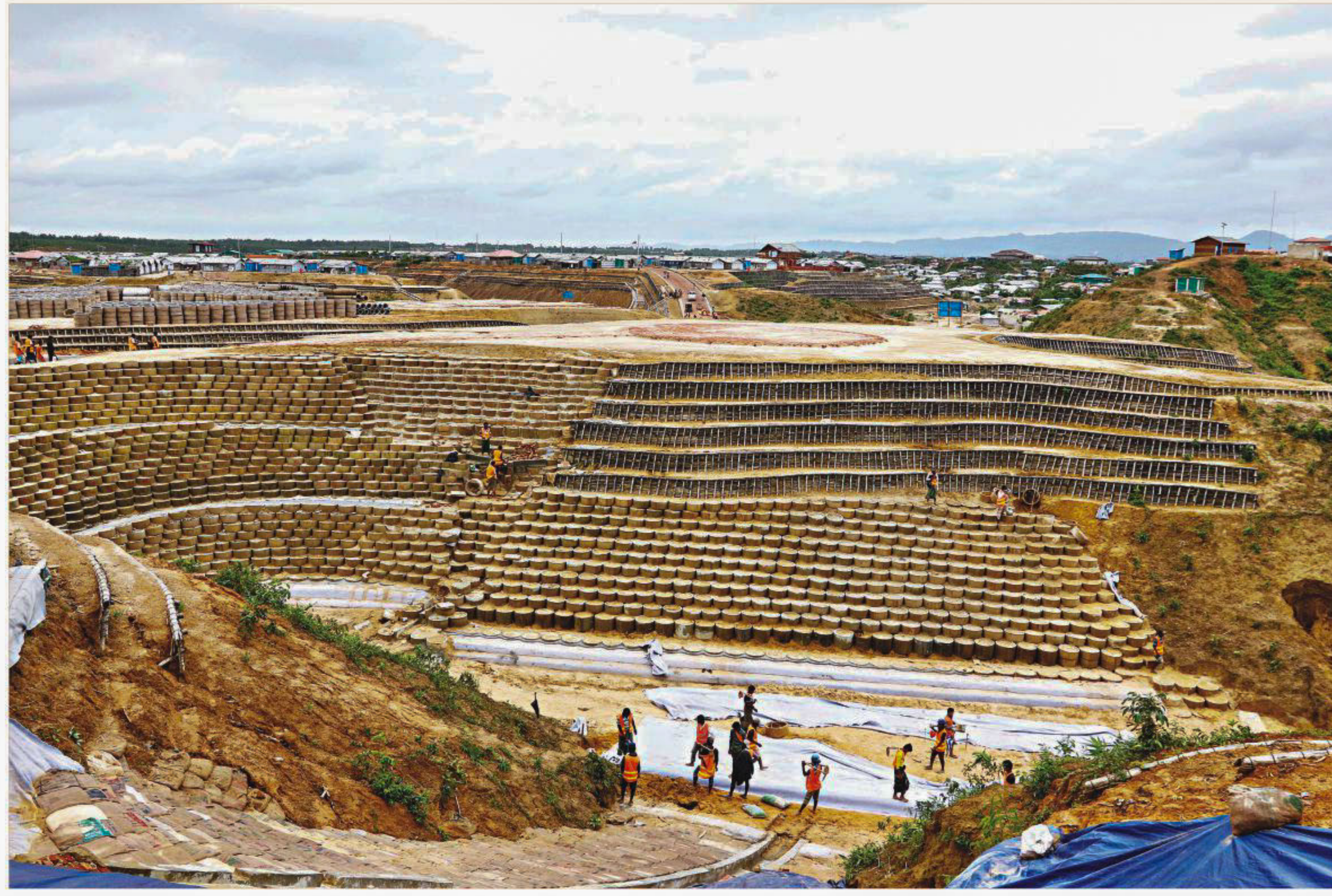
Once a lolling lush hillock alive with songs of birds, this knoll in Cox's Bazar's Balukhali is now anything but, thanks to its destruction for a Rohingya camp. This photo taken a couple of days ago shows thousands of concrete blocks and bamboos have been placed there to prevent landslide.
